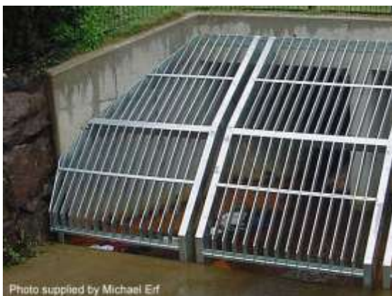
Parabolic inlet screen (Qld)
