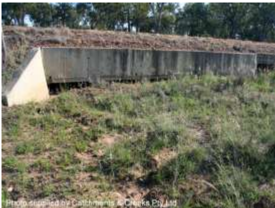
Blockage by clayey sediments (Qld)
