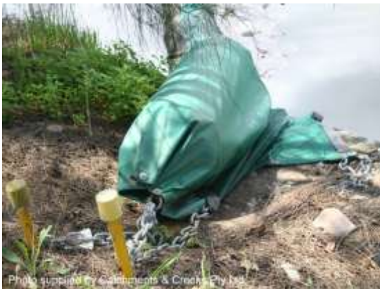
Anchor point for a floating curtain (NSW)
