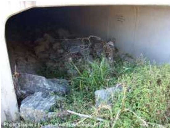
Blockage by boulders (Qld)
