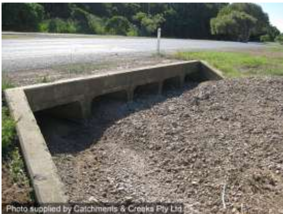
Blockage by gravel sediments (Qld)
