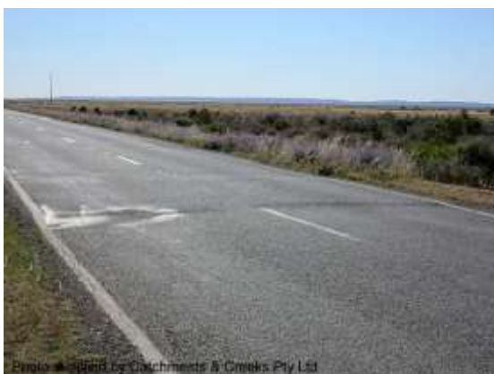
Lifting of pavement (Qld)
