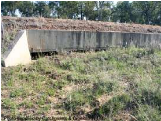
Severe sediment blockage (Western Qld)
