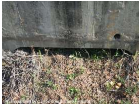
Blockage by clayey sediments (Qld)
