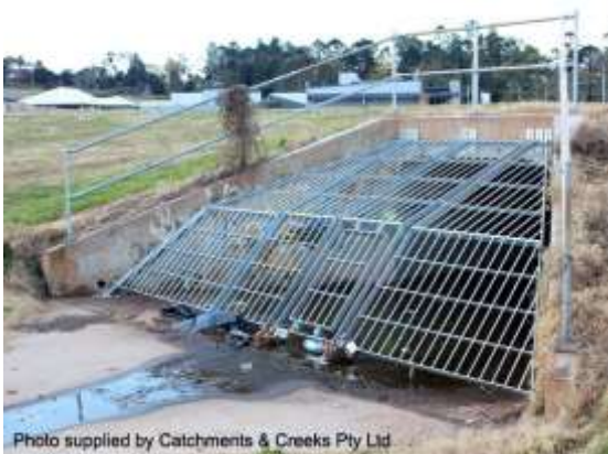
Parabolic inlet screen (Qld)
