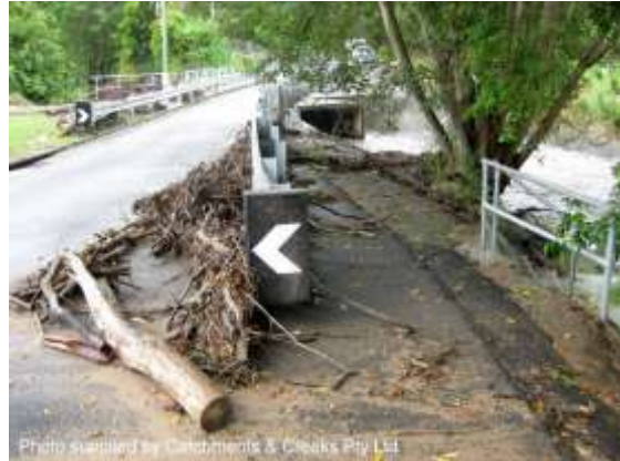
Debris trapped by traffic barriers (Qld)
