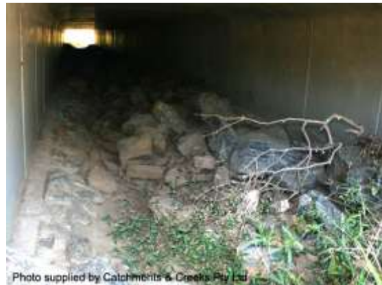
Blockage by boulders (Qld)
