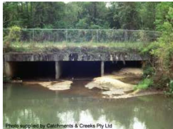
Blockage by sandy sediments (USA)
