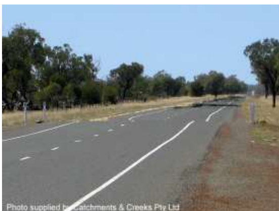
Lifting of pavement (Qld)
