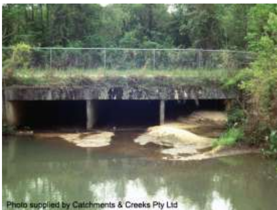
Deposition of sand in a culvert (USA)
