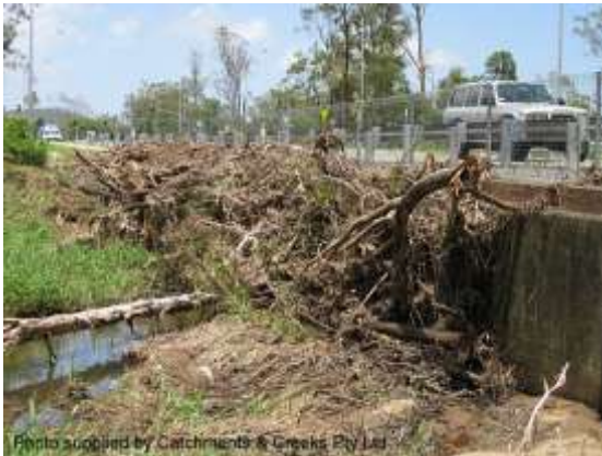
100% blockage of a road culvert (Qld)
