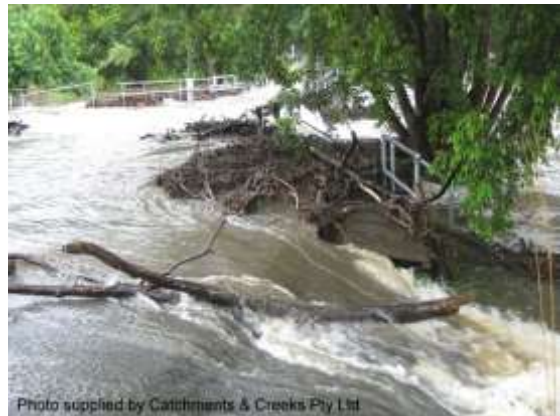
Debris trapped by traffic barriers (Qld)
