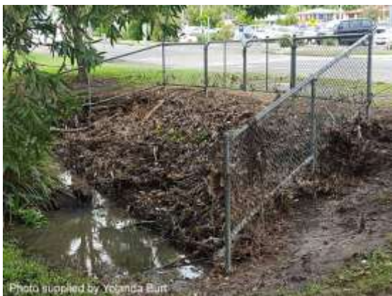
Fully blocked inlet screen (Qld)
