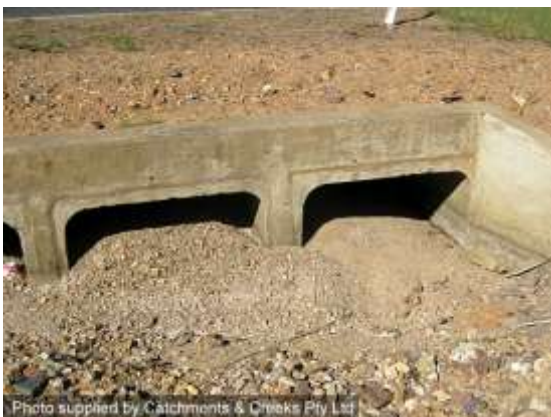
Partial sediment blockage of a culvert
