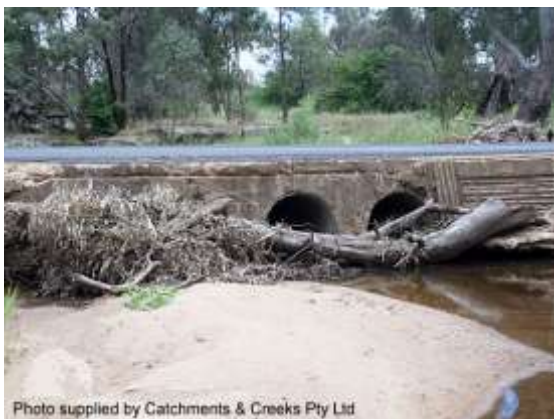
Log 'bridging' across the culvert inlet
