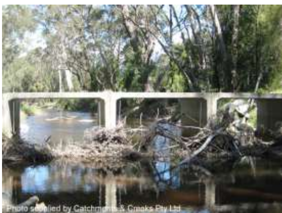
Partial blockage of a thin-deck culvert
