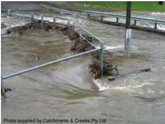
Debris trapped by handrails (Qld)
