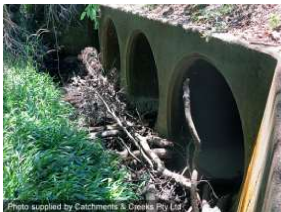
Debris blockage (Qld)
