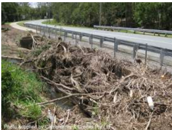
100 percent blockage of a culvert (Qld)
