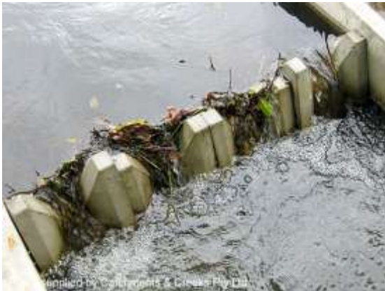
Debris blockage of fishway (Qld)
