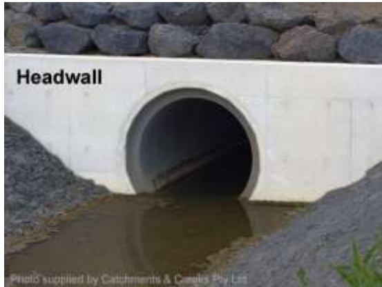
Culvert headwall without wingwalls
