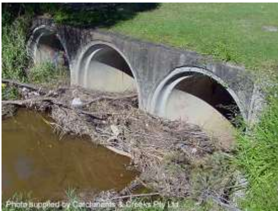
Low-level blockage of a road culvert
