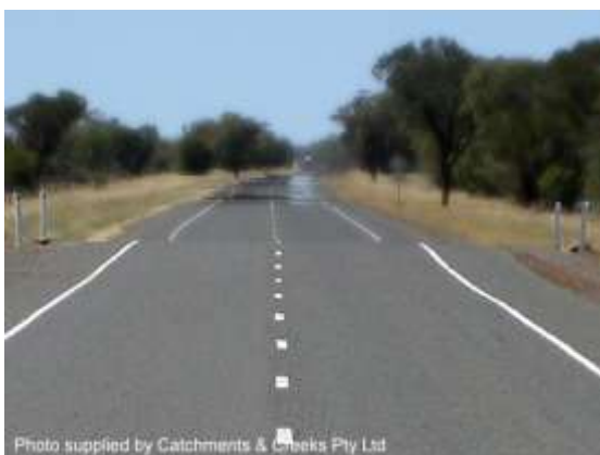
Lifting of pavement (Qld)
