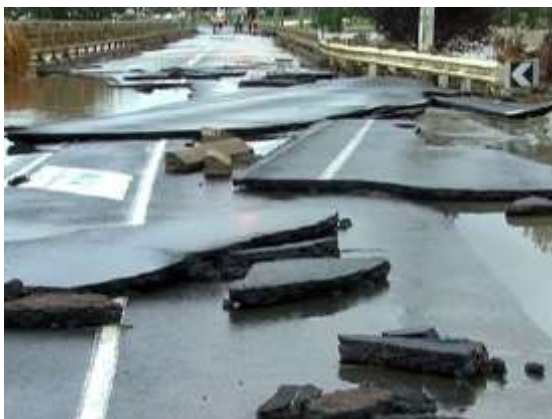
Road pavement lifted by floodwater (Qld)
