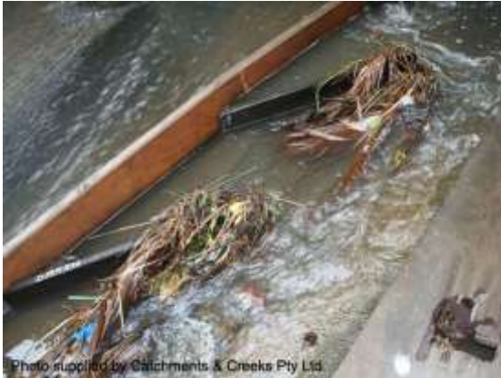
Debris caught on experimental baffles
