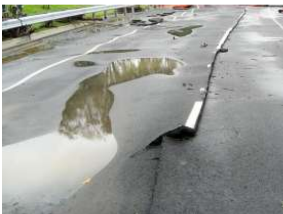
Displaced pavement (Qld)
