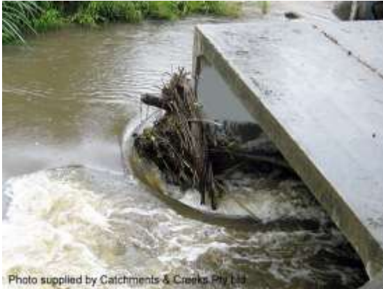
Debris wrapped around culvert legs (Qld)
