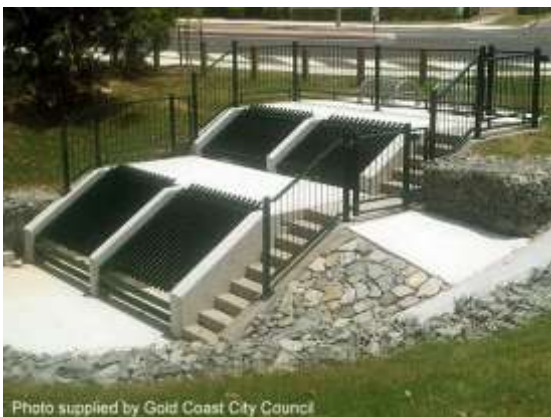
Complex inlet screen (Gold Coast, Qld)
