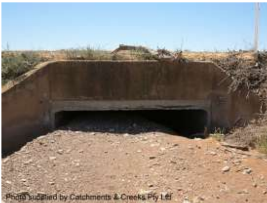
Sediment blockage of road culvert
