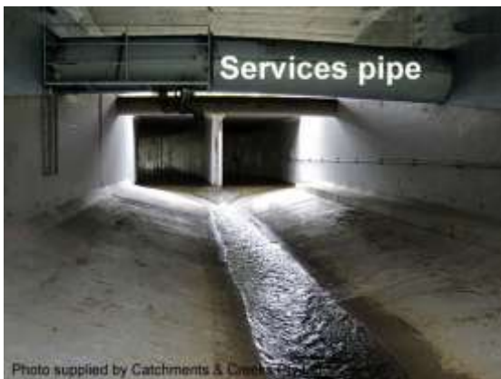
Culvert with exposed services (Qld)
