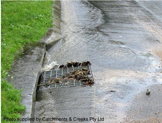
Roadside kerb drainage
