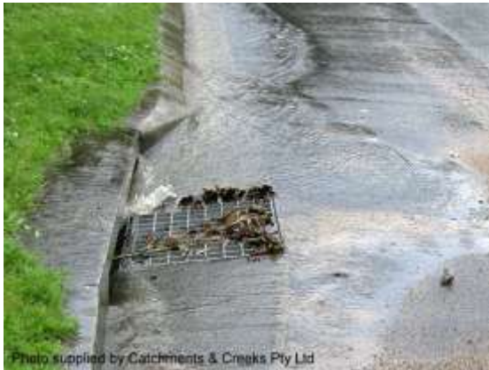
Photo supplied by Catchments & Creeks Pty Ltd Roadside kerb drainage
