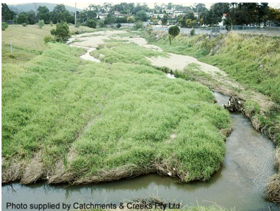
Sediment deposition in a widened channel
