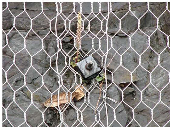
Rockfall netting (anchored to rock)
