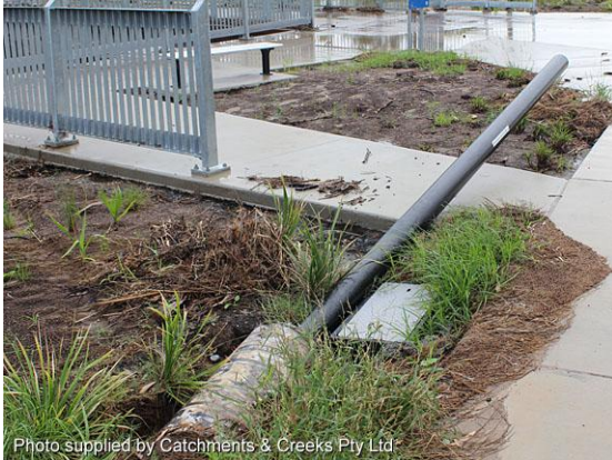
Damage to infrastructure (Qld)
