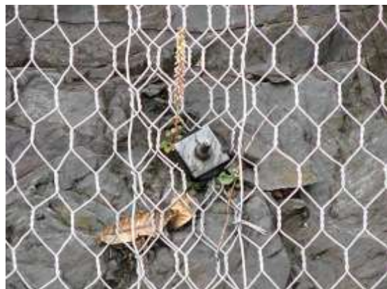
Rockfall netting (anchored to rock)
