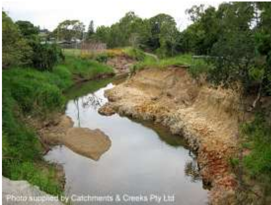
Bed and bank scour (Qld)
