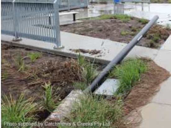
Damage to infrastructure (Qld)
