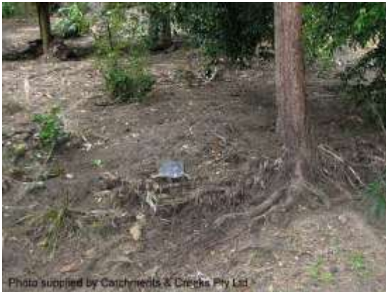
Soil scour following weed removal
