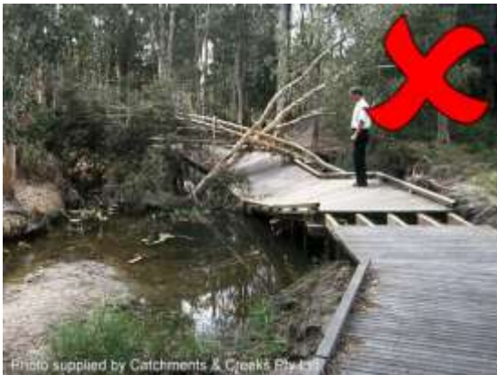
failed boardwalk crossing a creek
