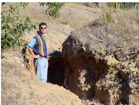
Lateral bank erosion (Qld)
