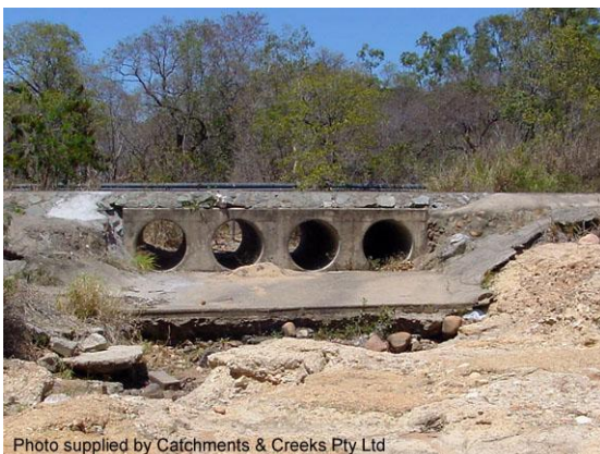
Bed level falling downstream of culvert
