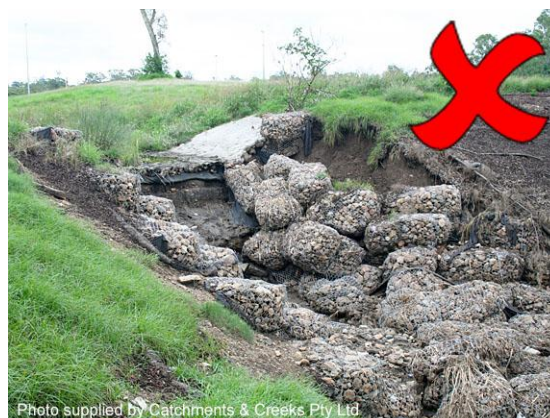
Gabion drop structure failure (Qld)
