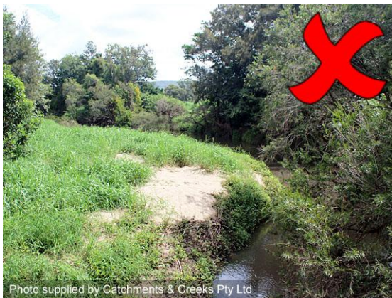
Sediment deposition in a widened creek
