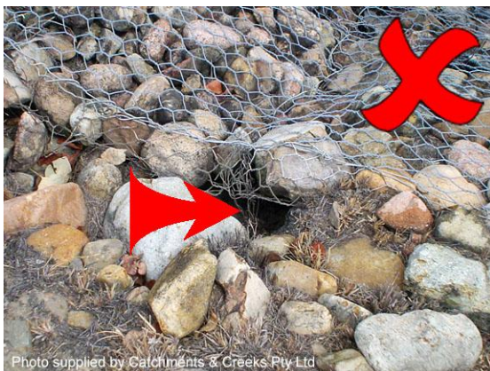
Tunnel erosion under a rock mattress
