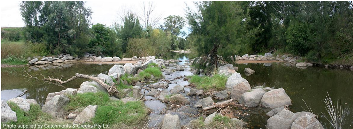
Rock ramp fishway looking downstream from the top of the fishway (Tamworth, NSW)
