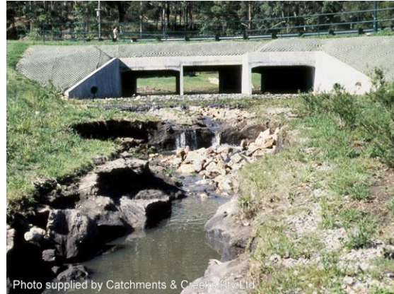
Failed placement of rock
