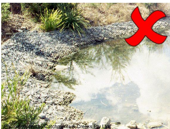
Mattress-lined sediment pond (Qld)
