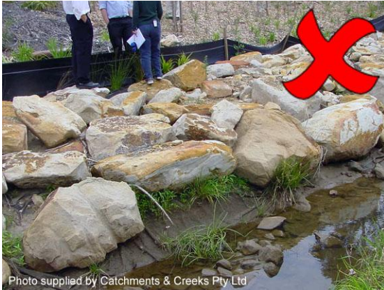
Undermining of toe rock
