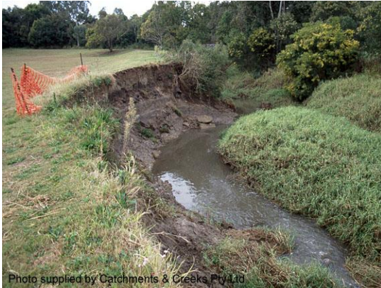
Bank scour (Qld)
