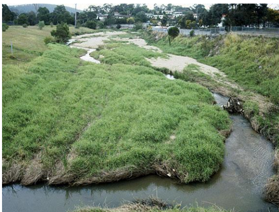
Sedimentation problems in a wide channel
