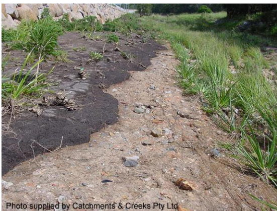
Flood damage to a grass-lined channel
