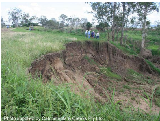
Bank slump (Qld)
