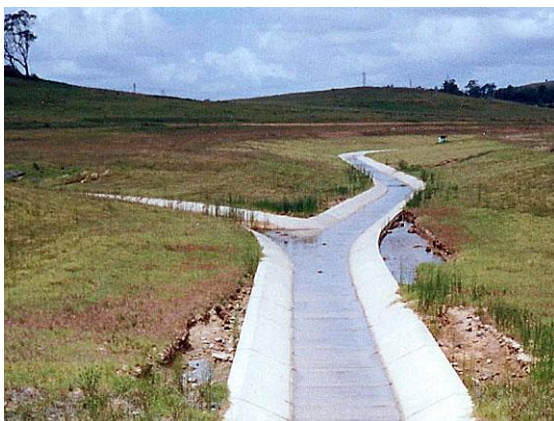
Post storm scour problem (NSW)
