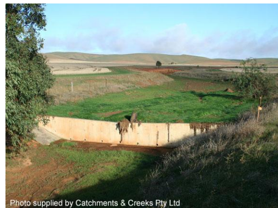
Vertical drop structure (SA)
