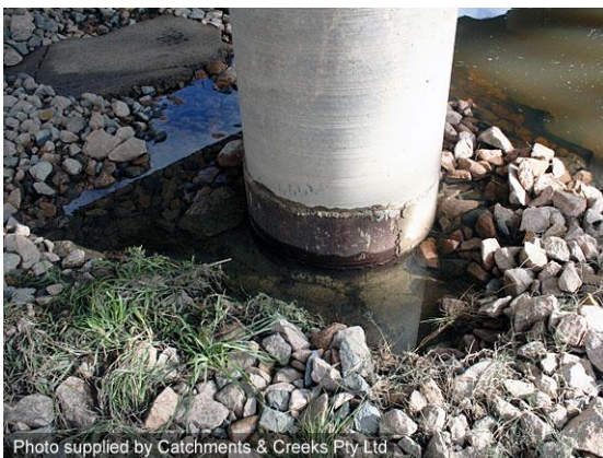
Scour around a bridge pier (Qld)
