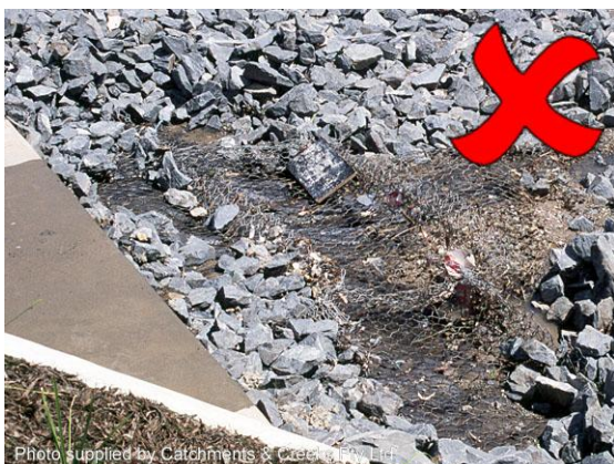
Stormwater outlet failure (Qld)
