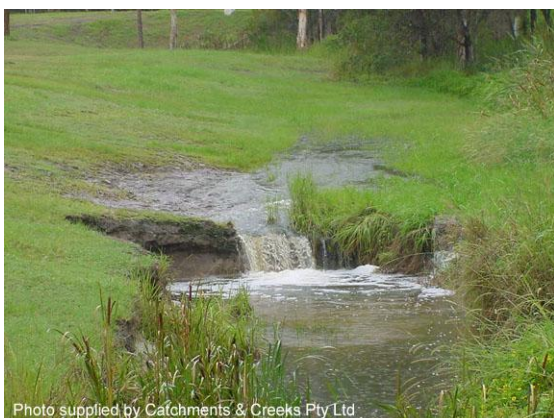
Formation of a scour hole (Qld)
