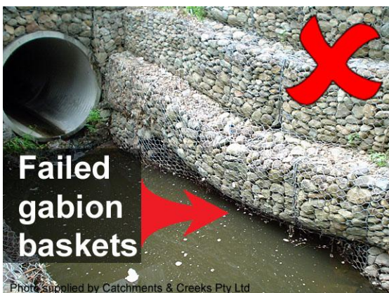
Stormwater outlet failure (NSW)
