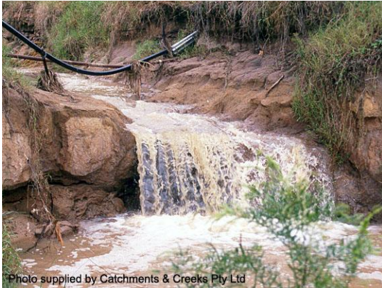
Soil scour (Qld)
