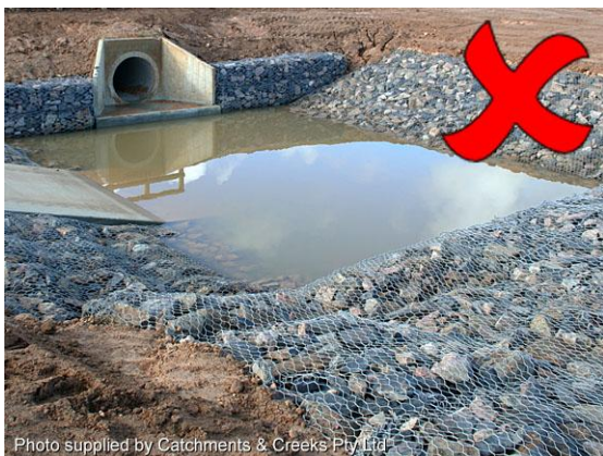
Mattress-lined sediment basin (SA)
