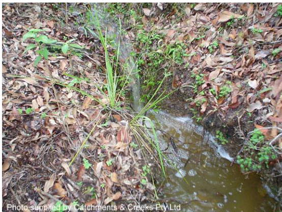
Scour along an overland flow path (Qld)
