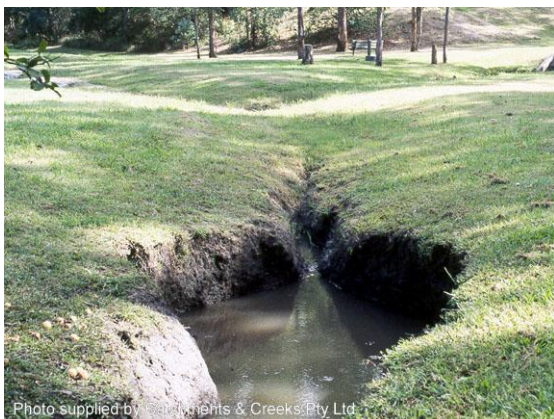
Scour along an overland flow path (Qld)
