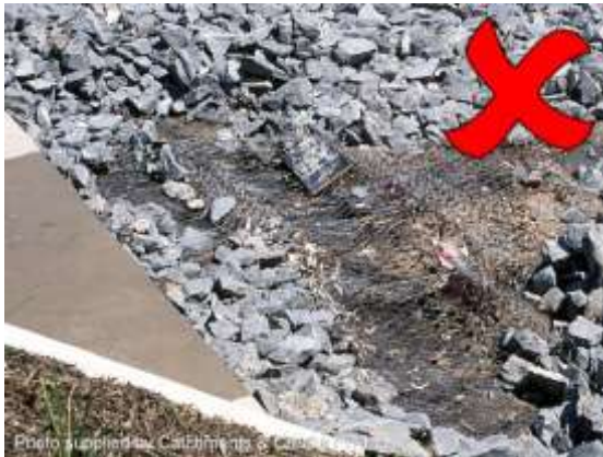
Stormwater outlet failure (Qld)
