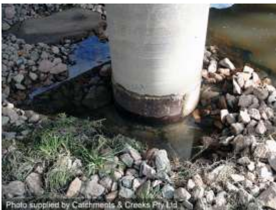
Scour around a bridge pier (Qld)
