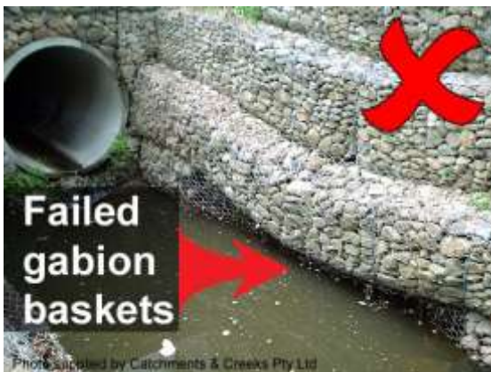
Stormwater outlet failure (NSW)
