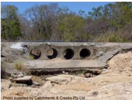
Bed level falling downstream of culvert
