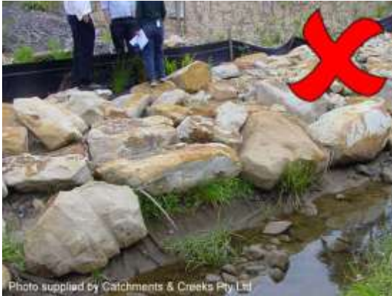
Undermining of toe rock
