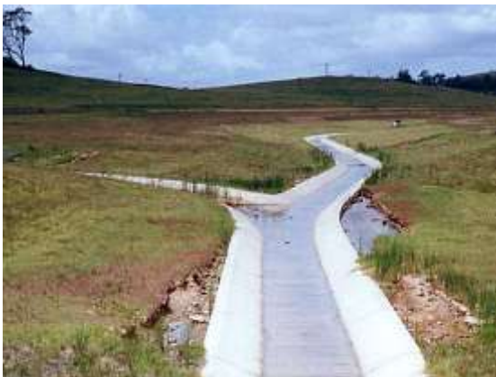
Post storm scour problem (NSW)
