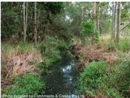
The above storm drain after plant growth
