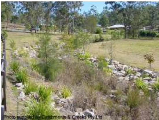
Vegetated drainage channel (Qld)
