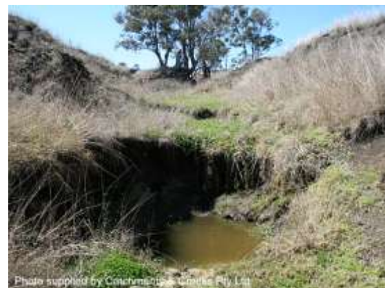
Scour along an overland flow path (Qld)
