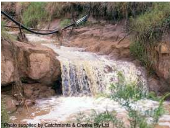
Soil scour (Qld)
