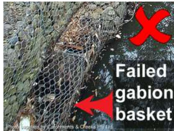
Failed basket in adjacent channel image
