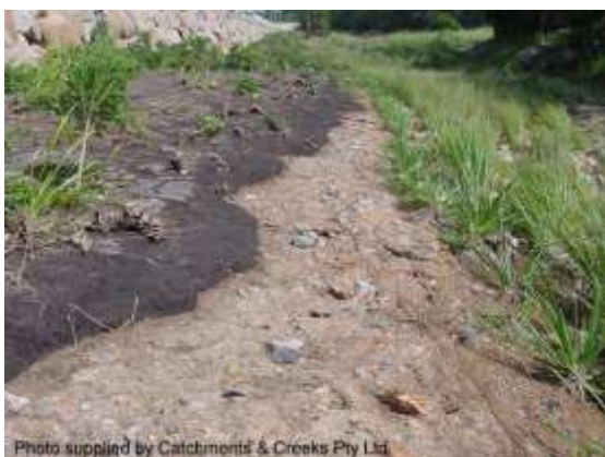
Flood damage to a grass-lined channel
