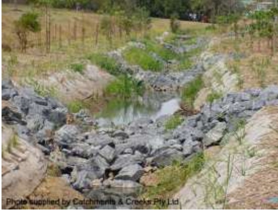
Benched storm drain (Qld)
