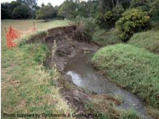
Bank scour (Qld)
