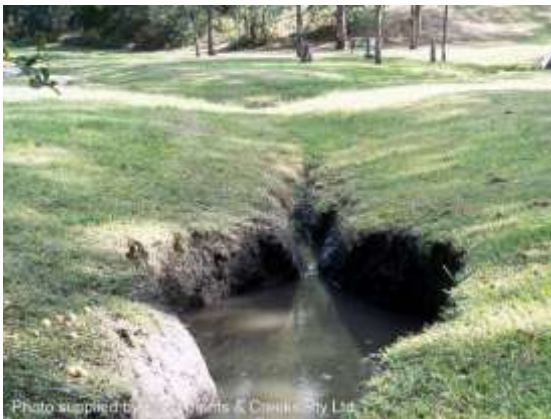
Scour along an overland flow path (Qld)
