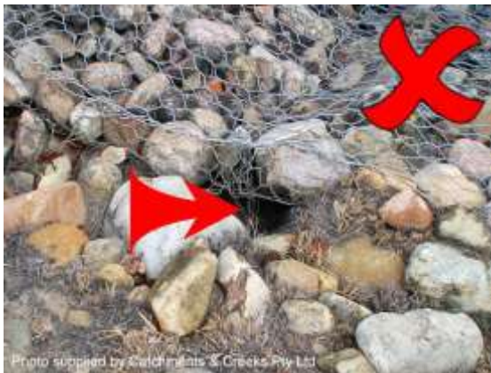
Tunnel erosion under a rock mattress
