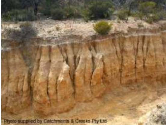
Fluting erosion in a dispersive soil (SA)
