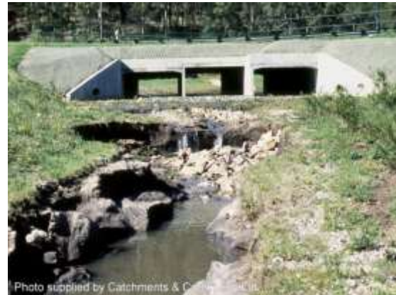
Failed placement of rock
