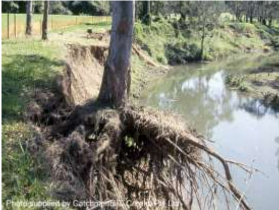
Exposed tree roots (Qld)
