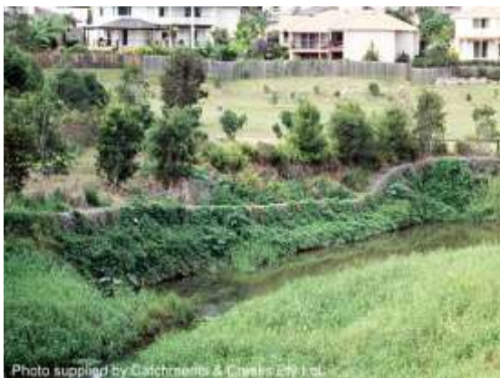
Vines and weeds cover gabions (Qld)
