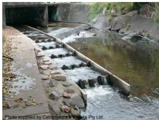
Precast concrete fishway (Qld)
