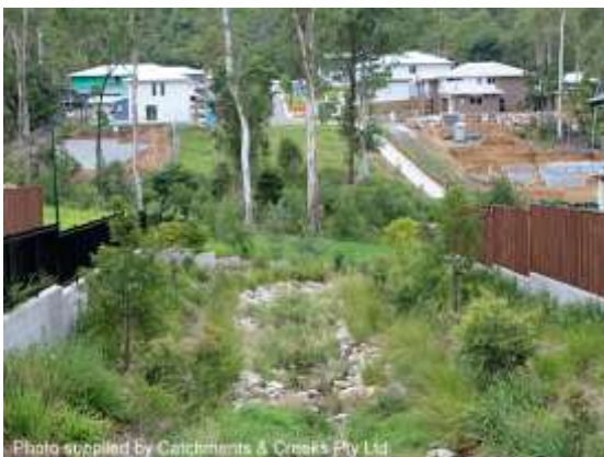
Vegetated drainage channel (Qld)
