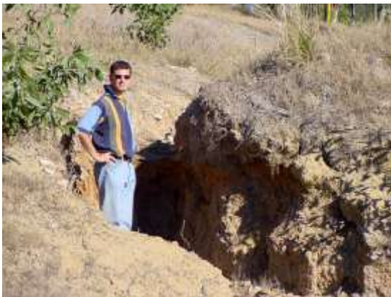
Lateral bank erosion (Qld)
