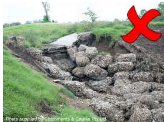
Gabion drop structure failure (Qld)
