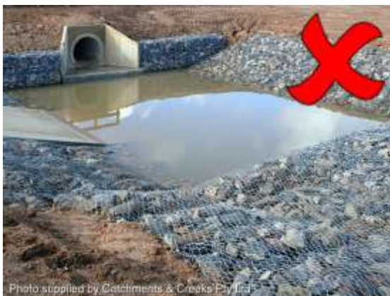
Mattress-lined sediment basin (SA)
