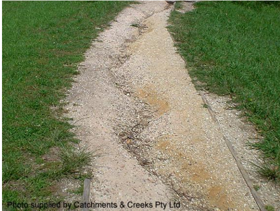
Rill erosion on a walking track (NSW)
