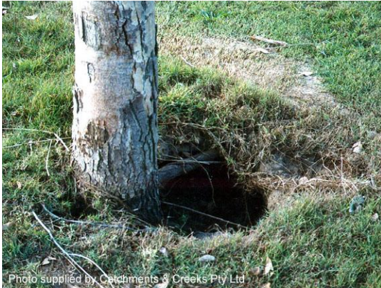
Flood-induced soil scour
