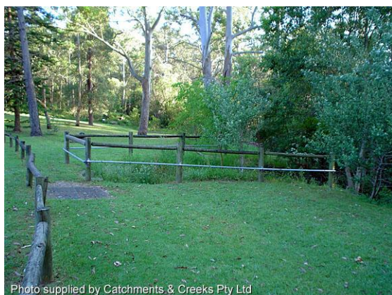
Recessed stormwater outlet (NSW)
