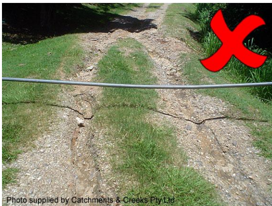
Soil erosion on an unsealed access road
