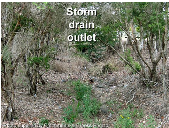
Vegetated minor storm drain (Qld)
