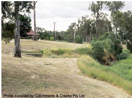
Recessed stormwater outlet (Qld)
