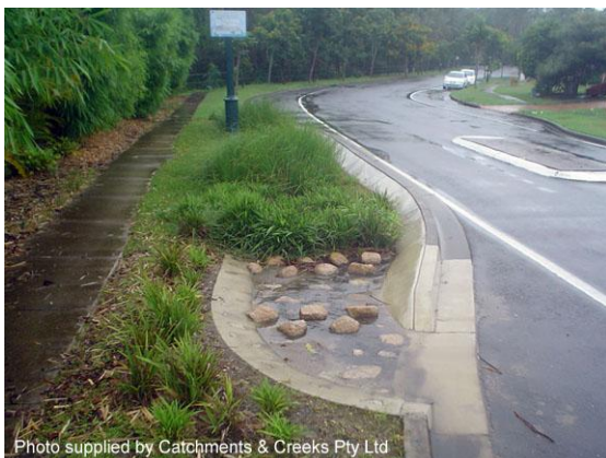
Stormwater filtration system (Qld)
