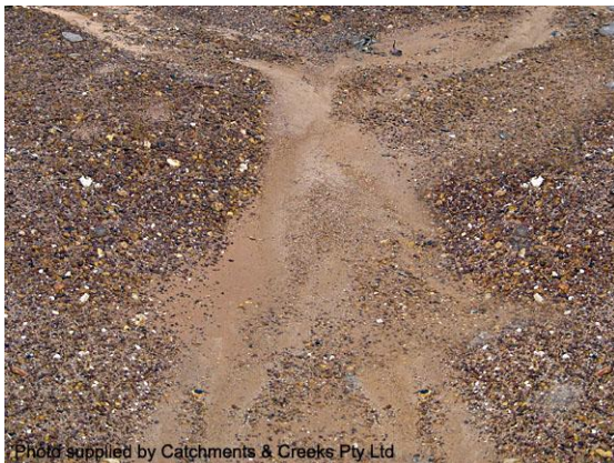
Eroded soil surface
