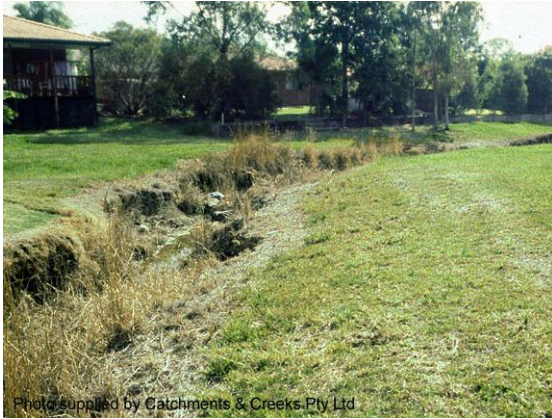
Storm drain without riparian vegetation
