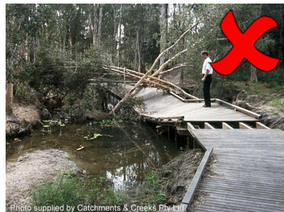
Flood damage to creek boardwalk
