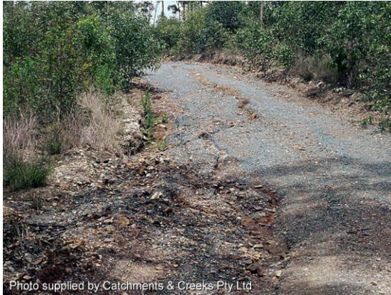
Water damage to an access road
