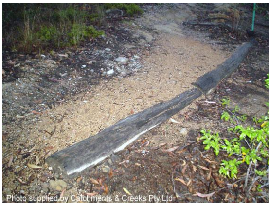
Recessed log check dam (cross bank)
