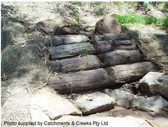
Discharge from a cross bank (NSW)
