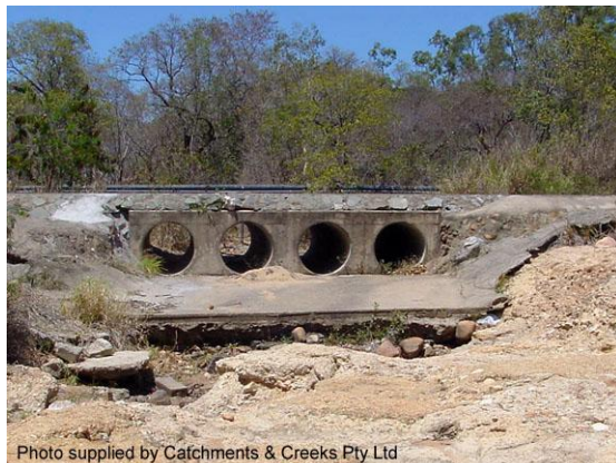
Bed level falling downstream of culvert
