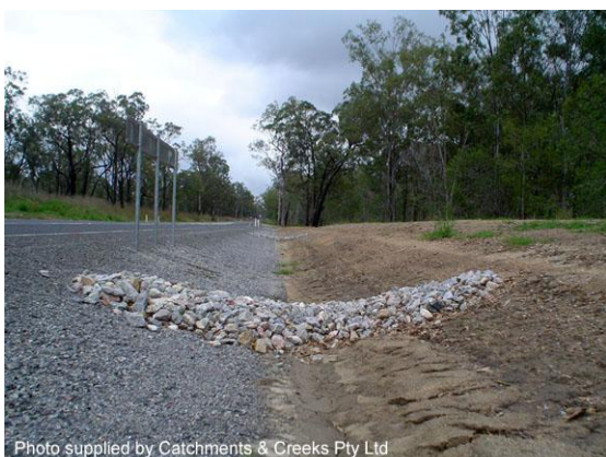
Rock check dam (Qld)
