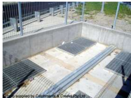
Skylights placed within the median (Qld)
