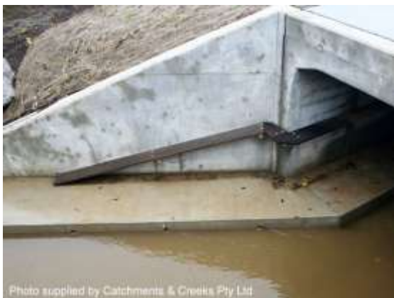
Box culvert with terrestrial pathways (Qld)
