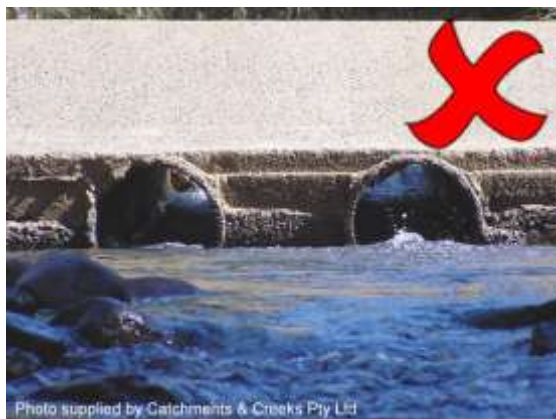
High-velocity, low-flow pipes
