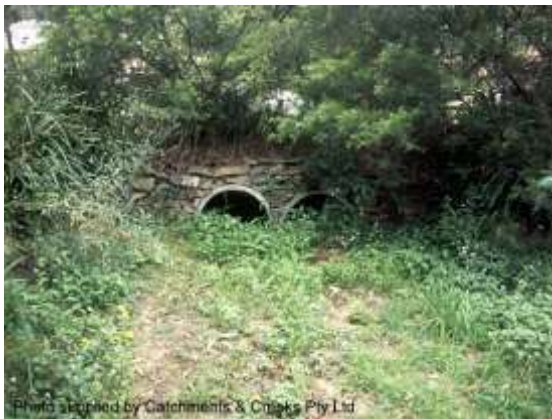
Recessed stormwater outlet (Qld)
