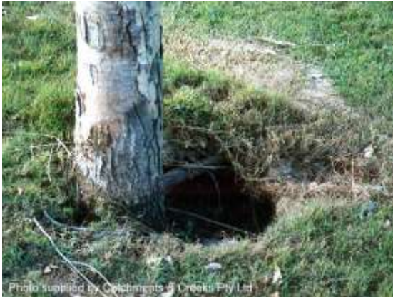
Flood-induced soil scour
