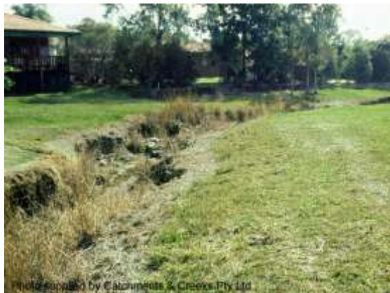
Storm drain without riparian vegetation
