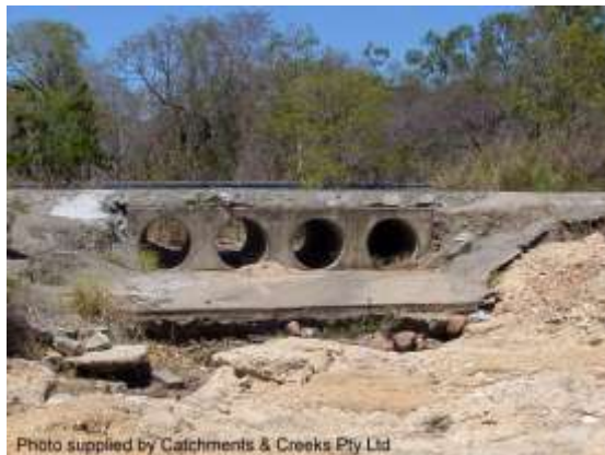
Bed level falling downstream of culvert
