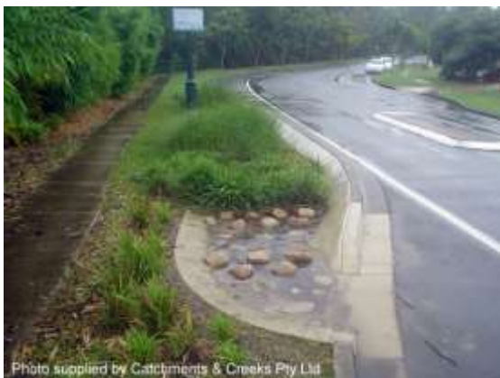
Stormwater filtration system (Qld)
