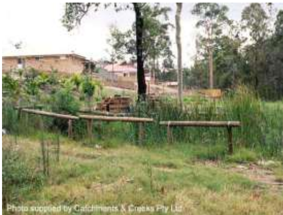
Recessed stormwater outlet (Qld)
