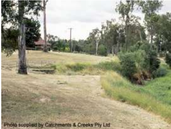
Recessed stormwater outlet (Qld)
