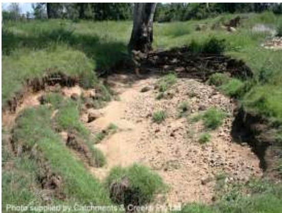
Erosion downstream of a floodplain tree
