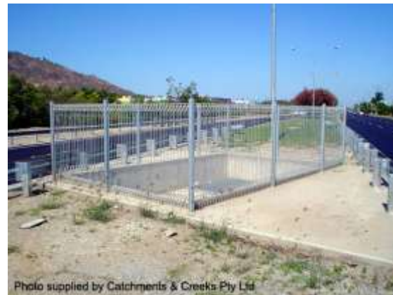
Skylights placed within the median (Qld)
