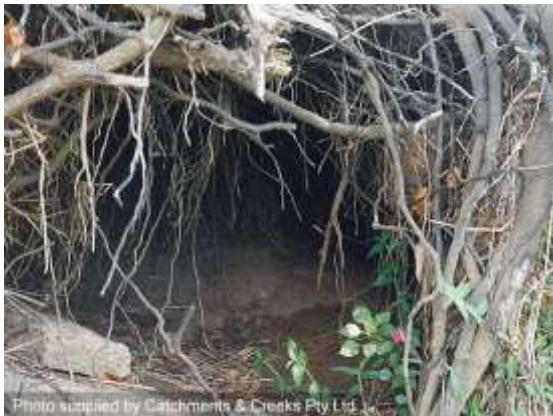
Undercut creek bank (Qld)
