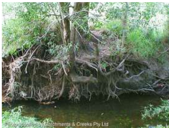
Undercut creek bank (Qld)
