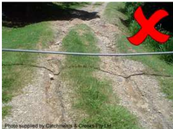
Soil erosion on an unsealed access road
