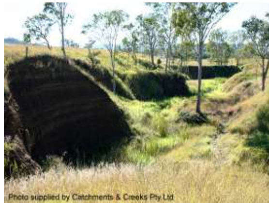
Bank slumping along the north bank (Qld)
