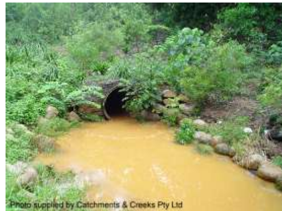
Recessed stormwater outlet (Qld)
