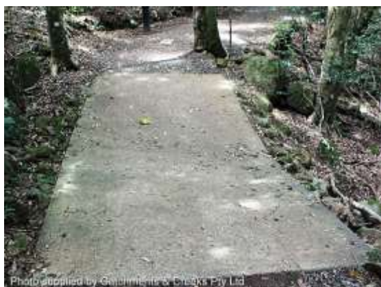
Photo supplied by Catchments & Creeks Pty Ltd Concrete cross drain on a walking track
