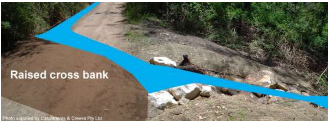
Outfall cross bank, which releases the flow down a stabilised rock-lined chute (NSW)
