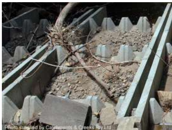
Sediment deposition within a fishway
