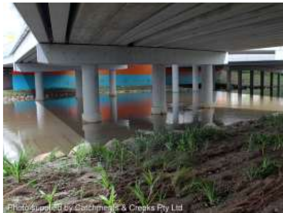
Plants shaded from rainfall under a bridge
