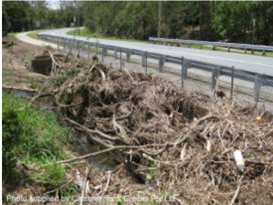
Debris blockage of culvert entrance
