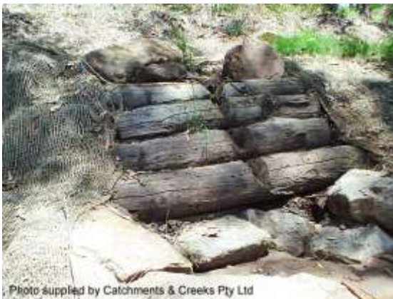
Discharge from a cross bank (NSW)
