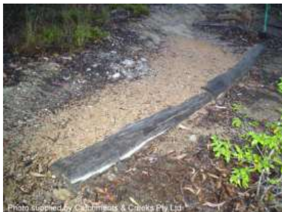
Recessed log check dam (cross bank)
