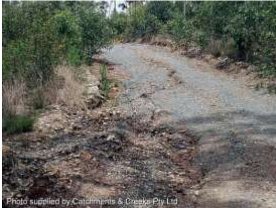
Water damage to an access road
