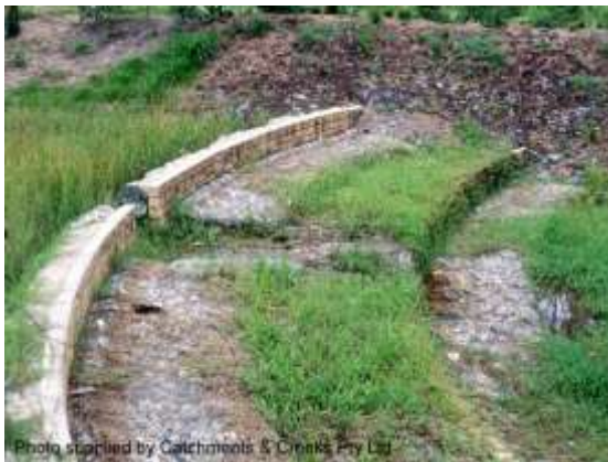
Stepped rock-mattress drop structure (Qld)
