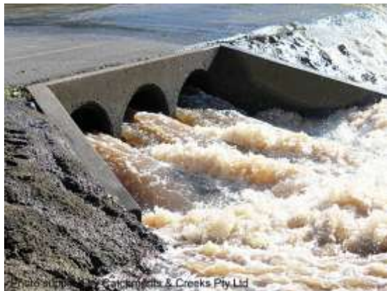
Excessive flow velocities (Qld)
