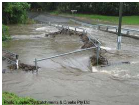
Floodwater overtop a road culvert
