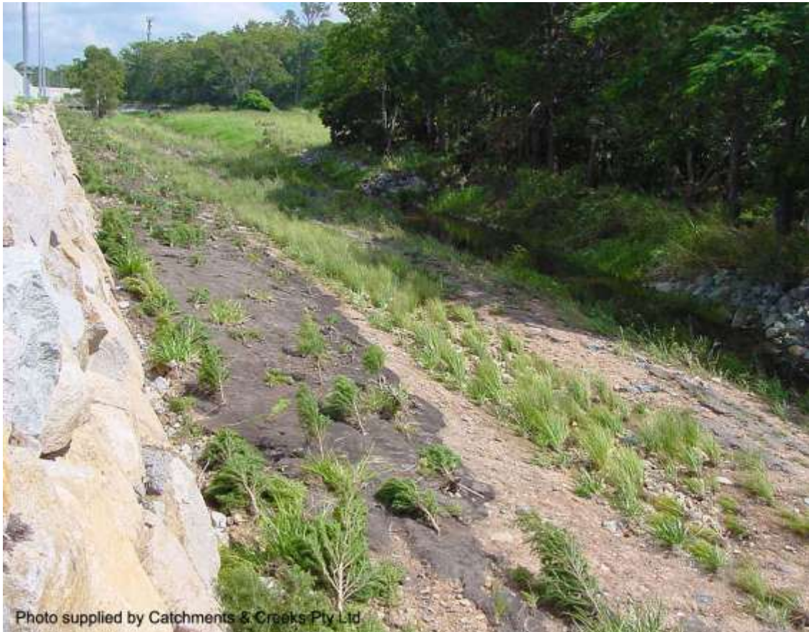
Looking downstream towards the culvert (after flood damage, 2001)
