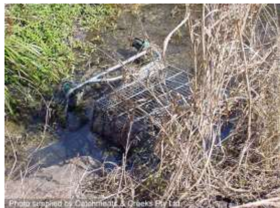
Deposition of rubbish in storm drain
