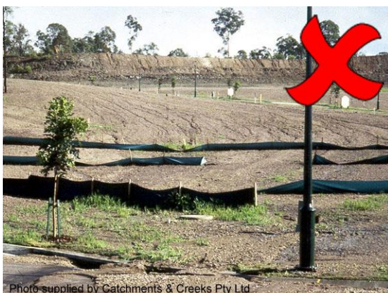
Inappropriate use of sediment fences
