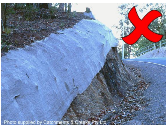
Poorly applied blanket
