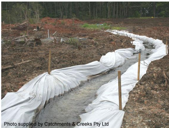
'Clean' water diversion drain
