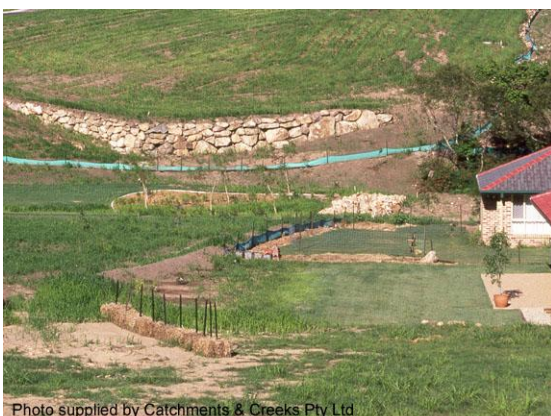
Straw bales diverting stormwater runoff
