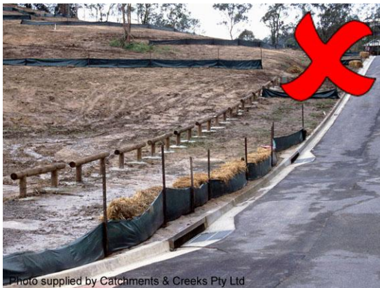
Inappropriate use of a sediment fence
