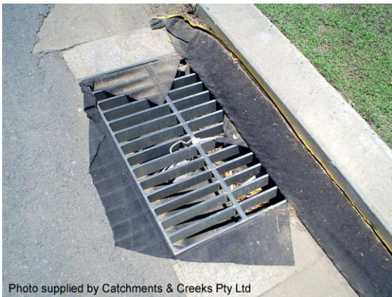
Gully bag sediment trap
