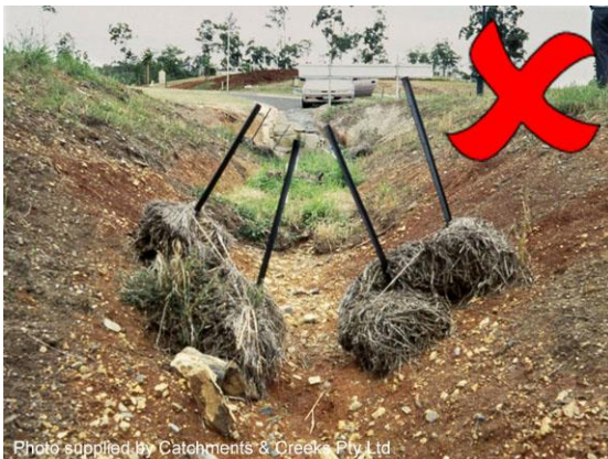
Failed straw bale sediment trap
