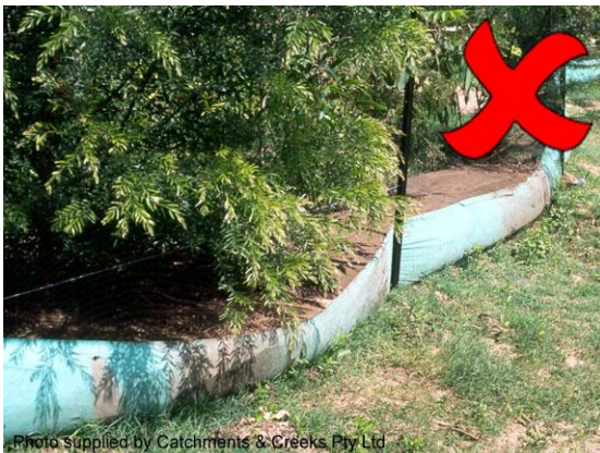
Sediment fence in need of maintenance
