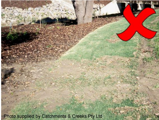
Evidence of concentrated runoff
