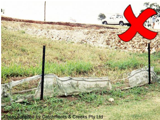
Sediment fence well past its 'use-by' date
