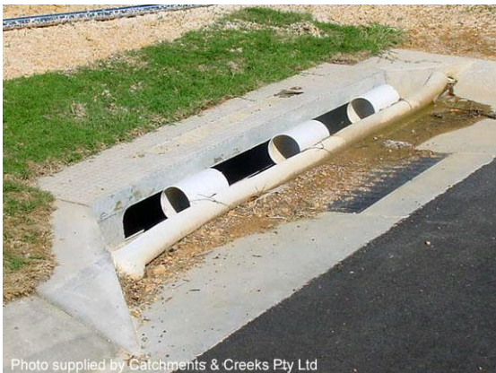
Sag inlet sediment trap
