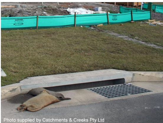
On-grade kerb inlet sediment trap
