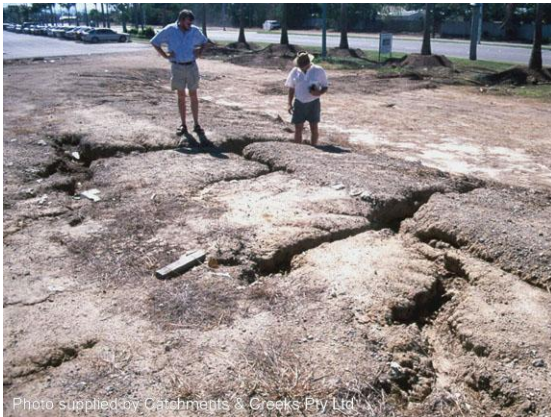
Inspecting storm damage
