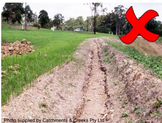
Erosion along channel invert
