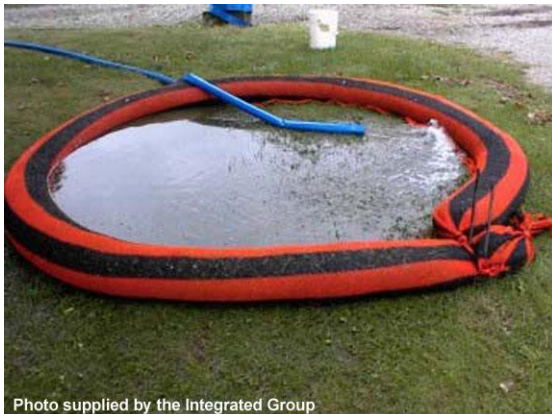
Compost-filled filter sock
