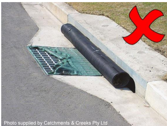
Poorly-design sag inlet protection
