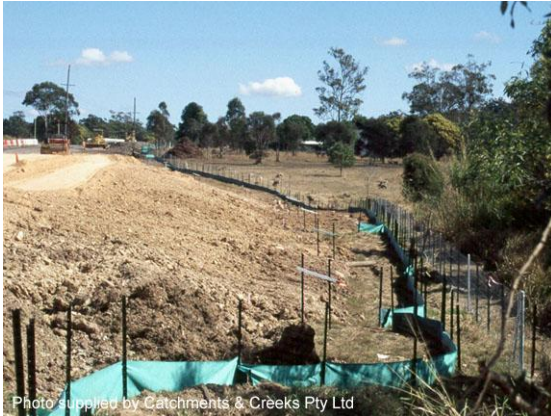
Sediment fence with regular 'returns'
