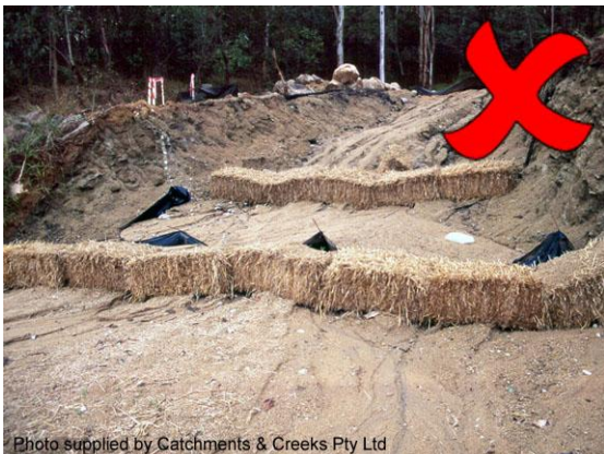
Inappropriate controls on a steep slope
