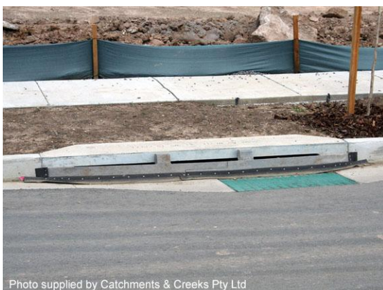
On-grade kerb inlet
