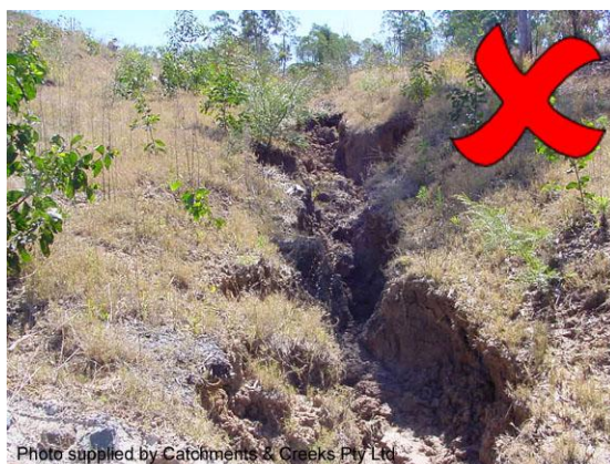
Failed diversion drain in a dispersive soil
