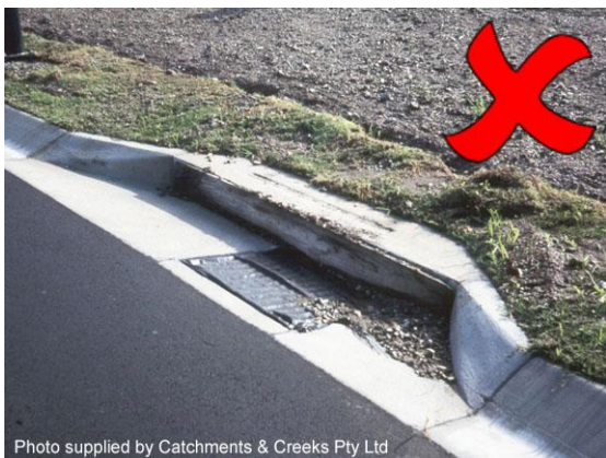
Fully blocked on-grade gully inlet
