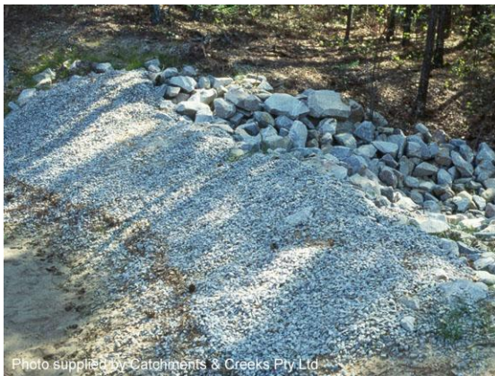
Rock filter dam with aggregate filter
