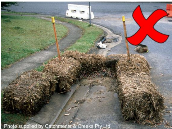
Potential traffic hazard
