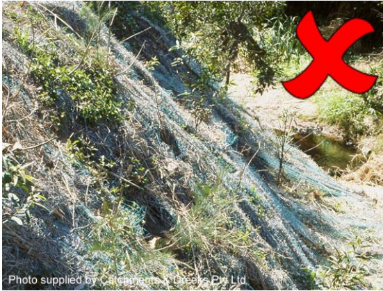
Misuse of synthetic blanket on creek bank
