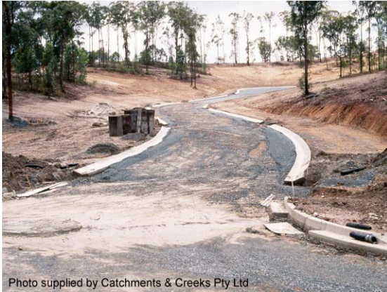
Erosion from a non-seasonal storm
