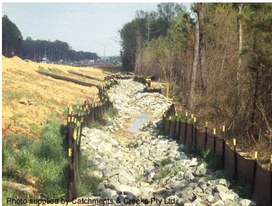
Protection of permanent storm drain
