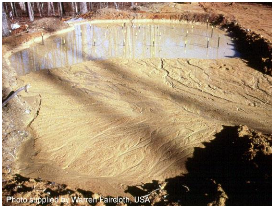
Sediment retained in a basin
