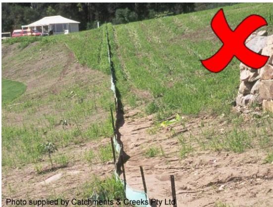
Inappropriate installation of a fence
