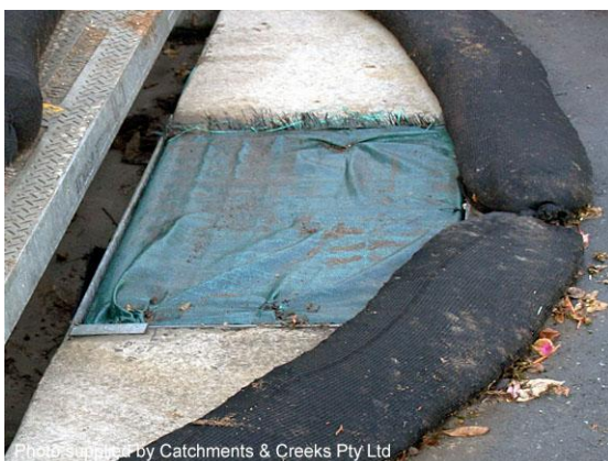
Inappropriate use of fabrics
