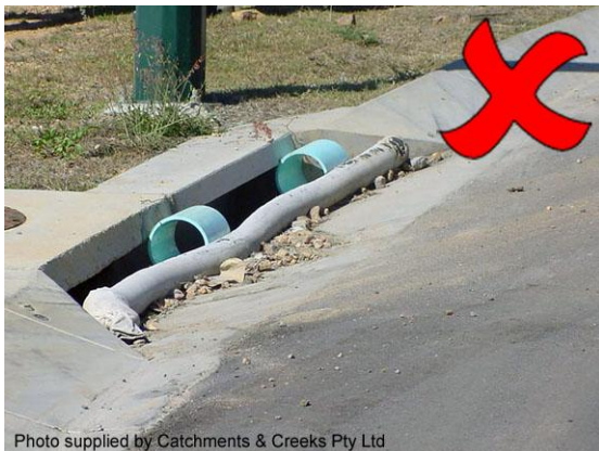
On-grade kerb inlet
