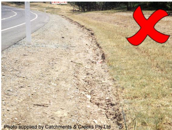
Rill erosion along edge of turf
