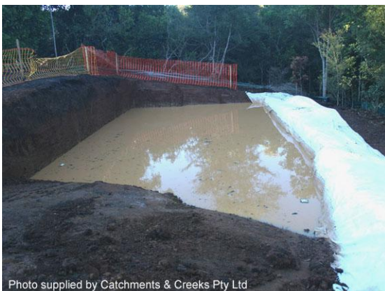
Basin full and ready to overflow
