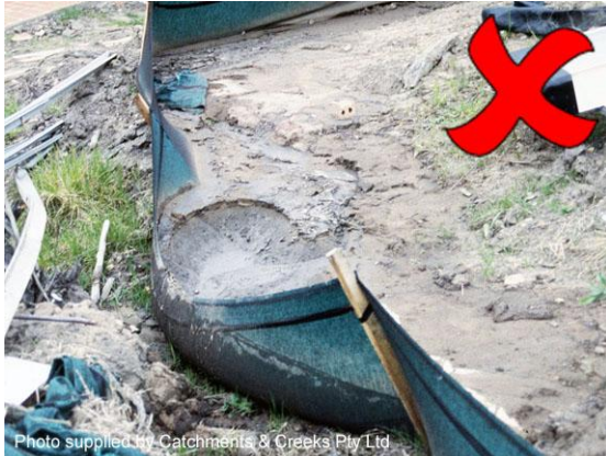
Sediment fence in need of maintenance
