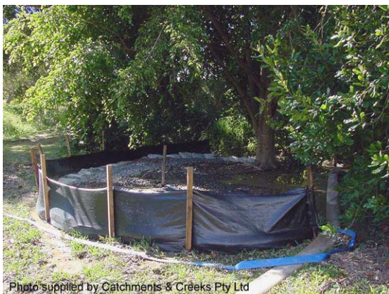
Off-stream filter pond
