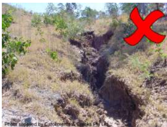
Failed diversion drain in a dispersive soil
