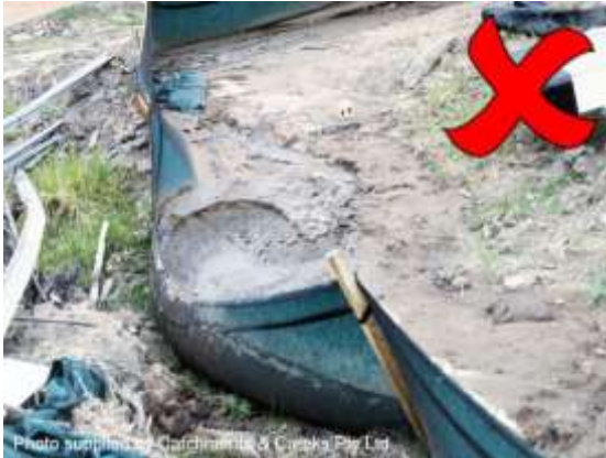
Sediment fence in need of maintenance
