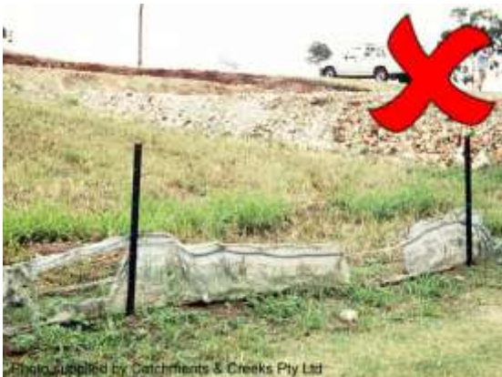
Sediment fence well past its 'use-by' date
