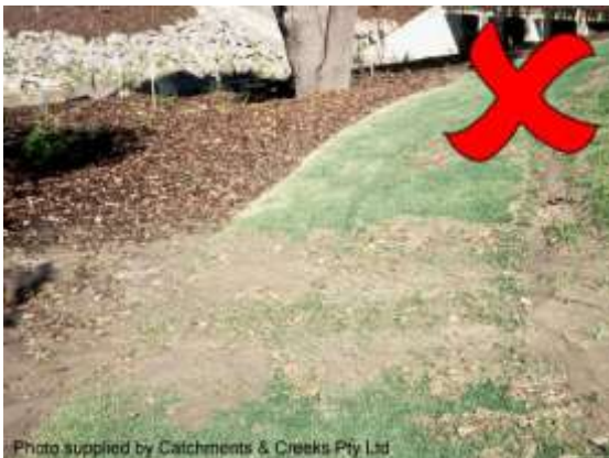
Evidence of concentrated runoff
