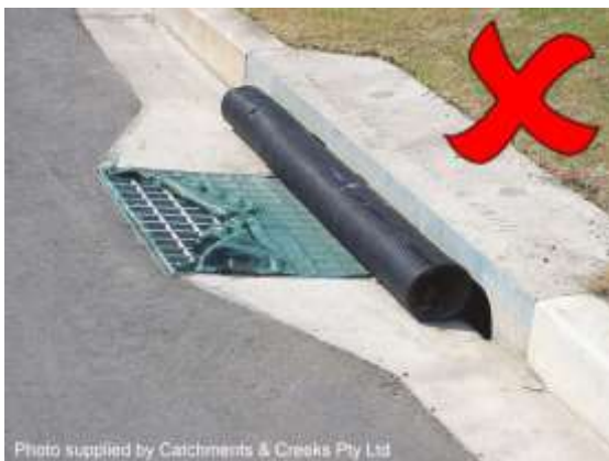
Poorly-design sag inlet protection
