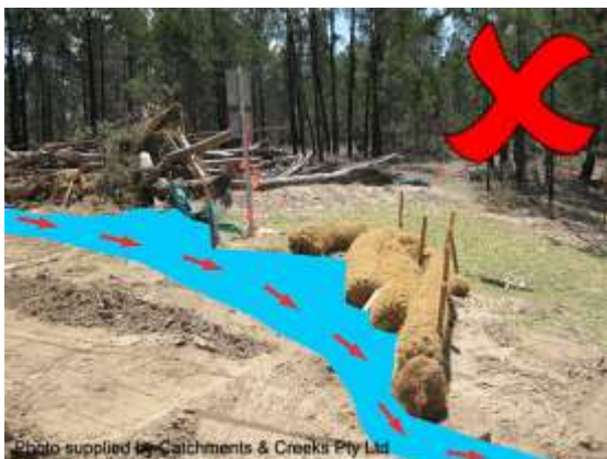
Stormwater runoff bypasses sediment trap
