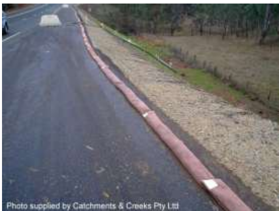
Temporary flow diversion system
