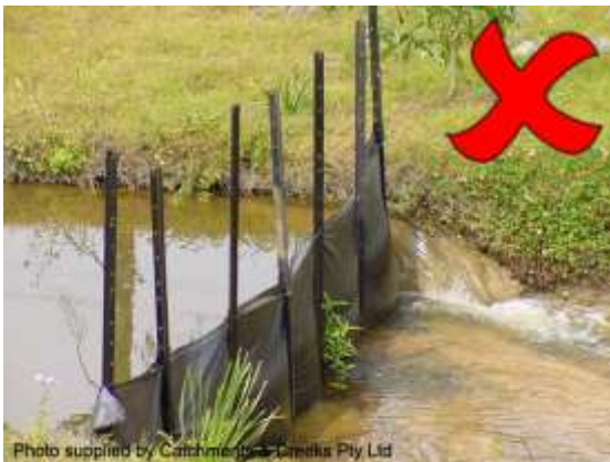
Poorly-designed sediment trap
