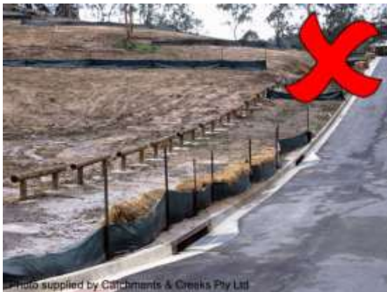
Inappropriate use of a sediment fence
