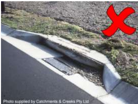
Fully blocked on-grade gully inlet
