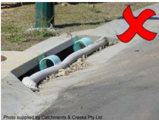
Fully blocked on-grade gully inlet
