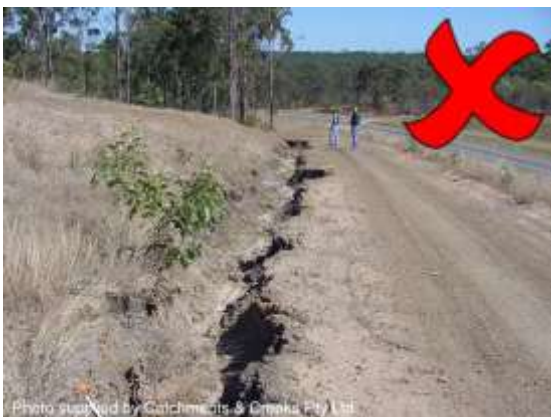
Batter drain cut into a dispersive soil
