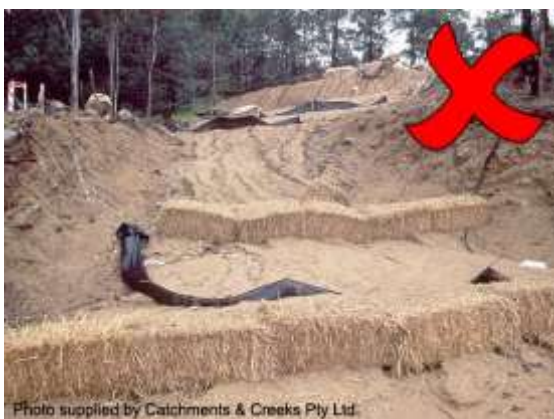
Failed sediment traps on a steep ramp
