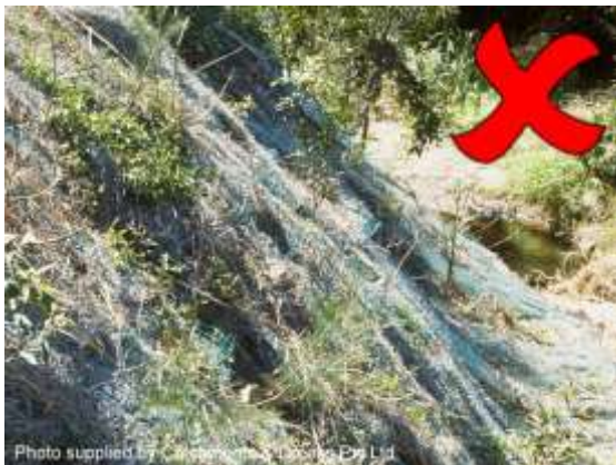
Misuse of synthetic blanket on creek bank
