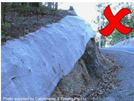
Poorly applied blanket
