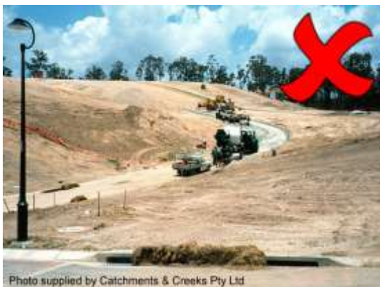
Excessive wet-season land clearing
