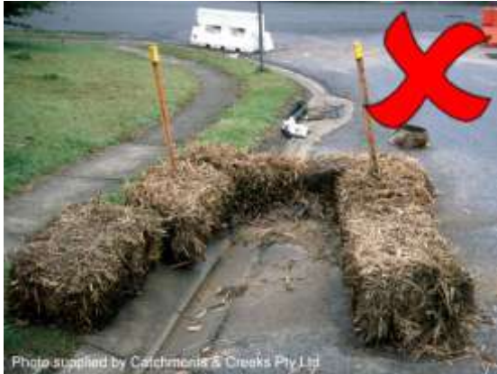
Potential traffic hazard
