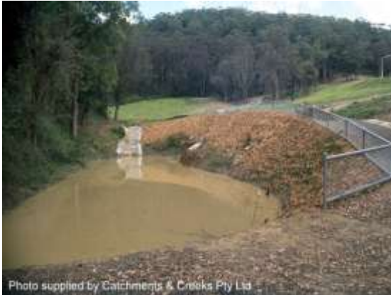
Basin with limited maintenance access
