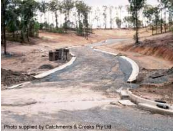
Erosion from a non-seasonal storm
