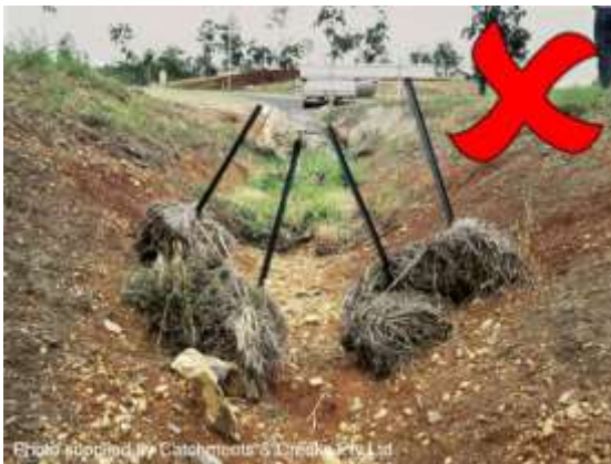
Failed straw bale sediment trap
