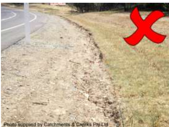
Rill erosion along edge of turf
