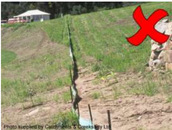
Inappropriate installation of a fence
