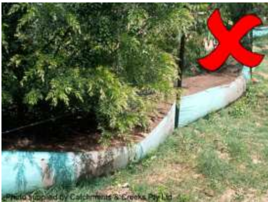
Sediment fence in need of maintenance
