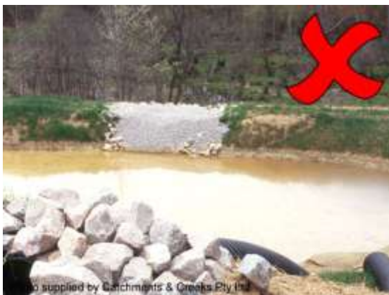
Poor sediment basin spillway design
