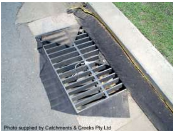
Gully bag sediment trap
