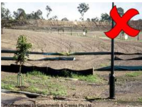
Inappropriate use of sediment fences
