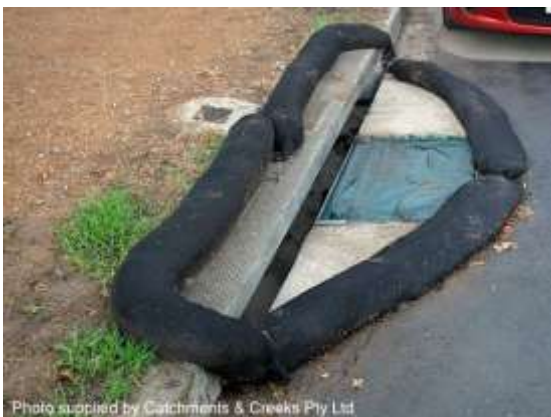
Sag inlet sediment trap
