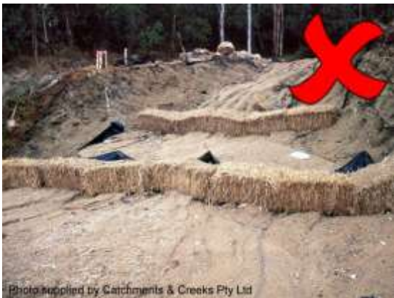
Inappropriate controls on a steep slope
