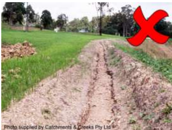
Erosion along channel invert
