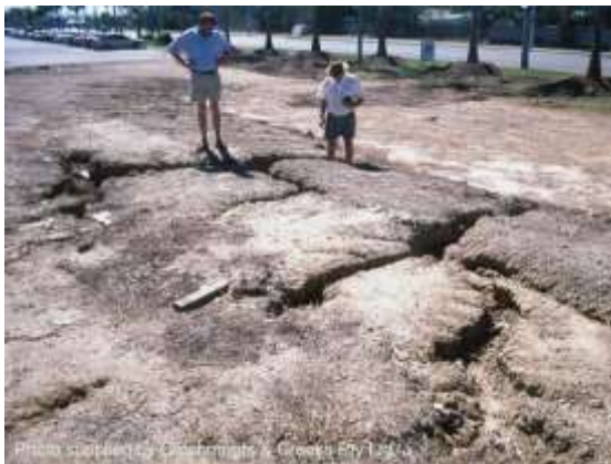
Inspecting storm damage
