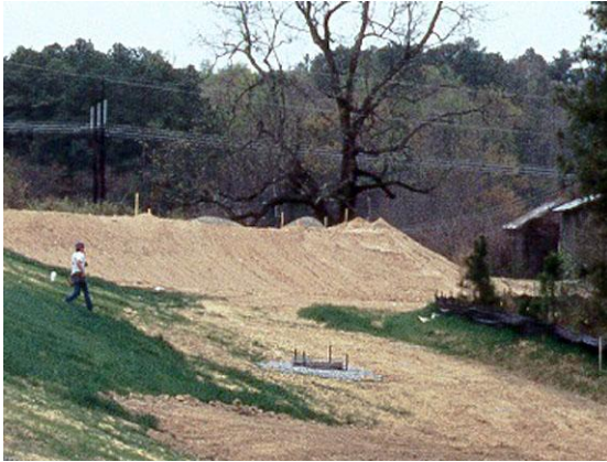
Drop inlet sediment trap (centre of image)
