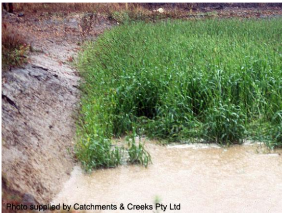
Very steep and slippery bank slope
