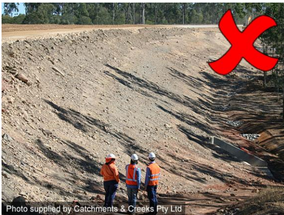
Batter without appropriate erosion control
