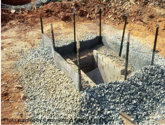
Mesh & aggregate drop inlet protection
