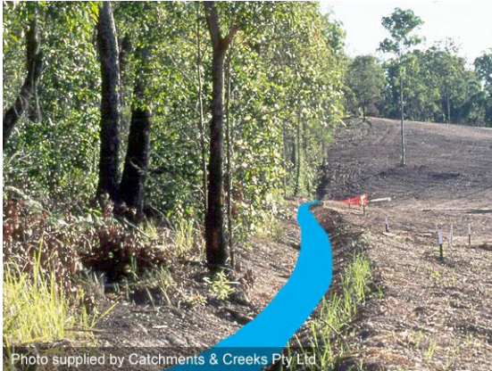
Photo supplied by Catchments & Creeks Pty Ltd Catch drain used to divert run-on water
