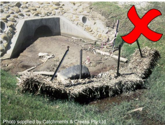
Inappropriate choice of sediment trap
