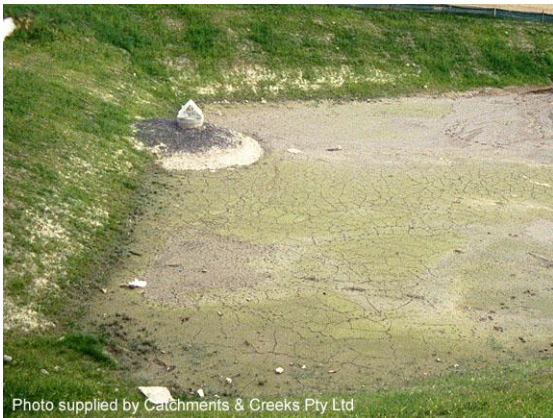
Type C sediment basin with grassed banks
