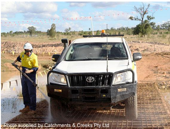
Vehicle wash-down area
