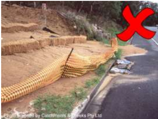
Sediment deposited off the site
