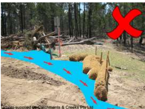
Stormwater runoff bypasses sediment trap
