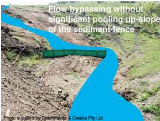
Sediment fence fails to capture sediment
