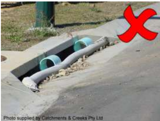
Inappropriate on-grade inlet control
