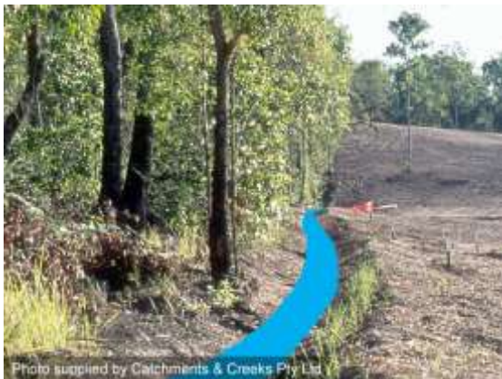
Catch drain used to divert run-on water
