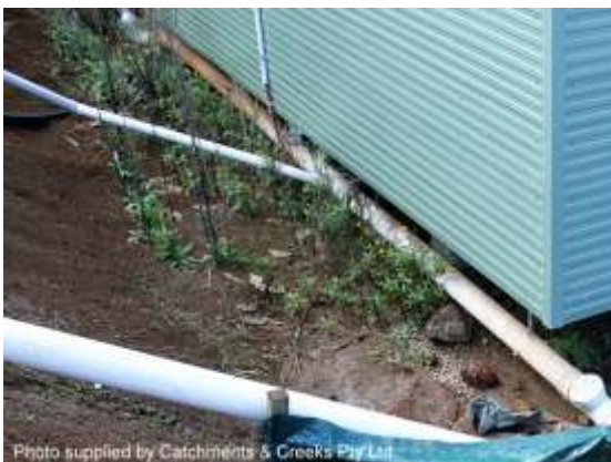
Temporary stormwater drainage
