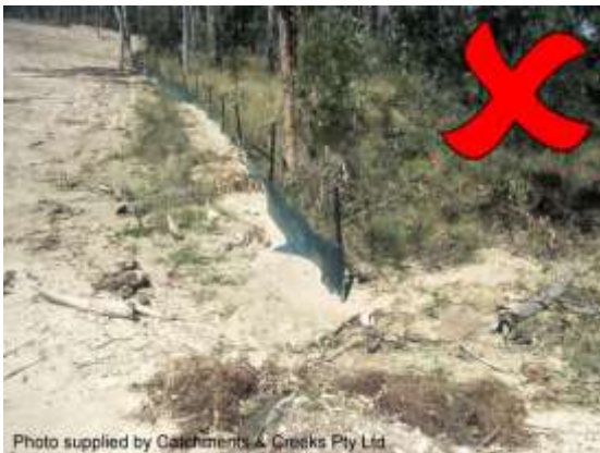
Fence not returned up-slope at end
