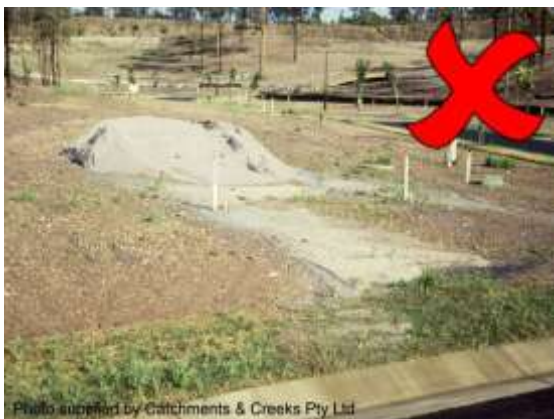
Stockpile locate on an overland flow path
