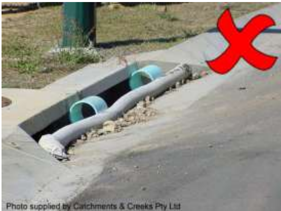
Common sense gone missing!
