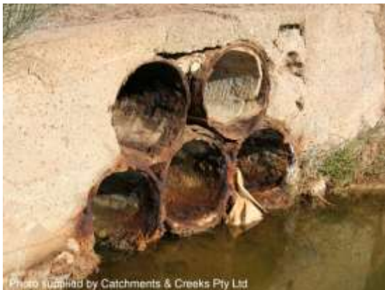
Culvert damaged by acidic water
