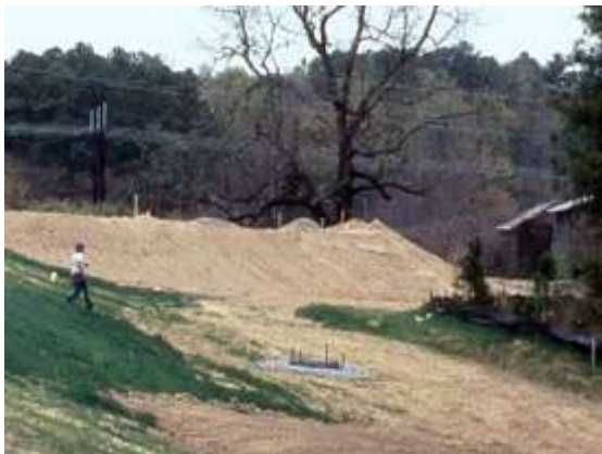
Drop inlet sediment trap (centre of image)
