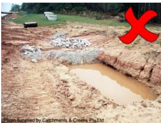
Sediment sump formed in dispersive soil
