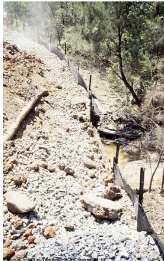
Spill-through weir & aggregate filter
