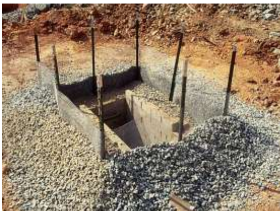
Mesh & aggregate drop inlet trap (1995)
