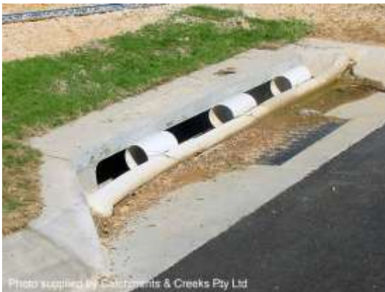
Sag inlet sediment trap
