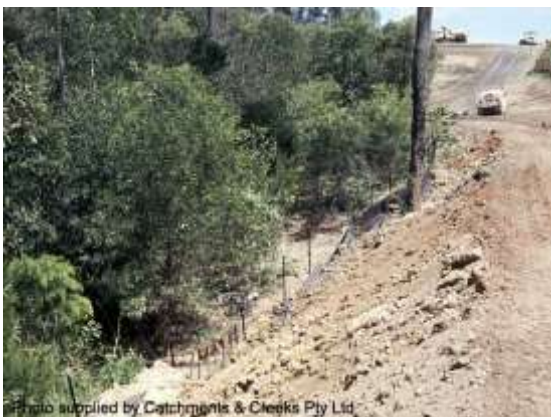
Spill-through weir outlet structure
