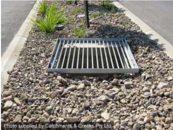
Field inlet located within median strip
