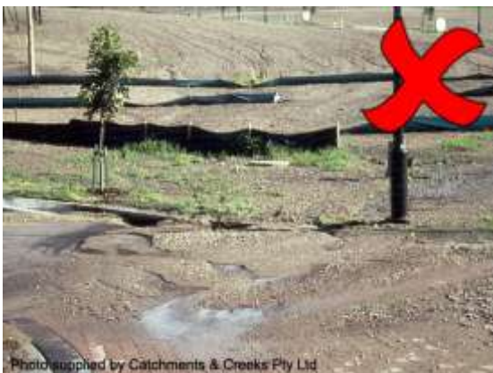
Inappropriate use of sediment fences
