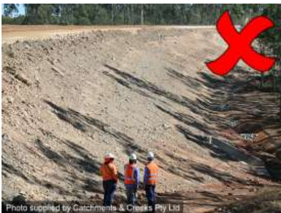
Batter without appropriate erosion control
