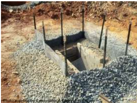
Mesh & aggregate drop inlet protection
