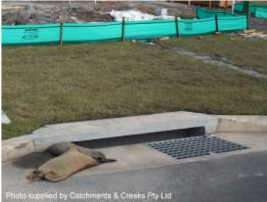
On-grade kerb inlet sediment trap
