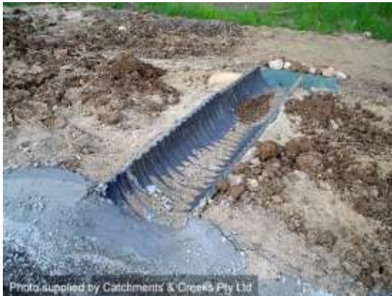
Temporary half-pipe batter chute
