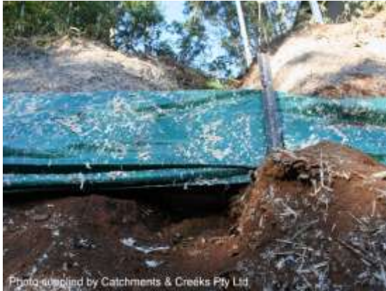
Storm undermines a sediment fence
