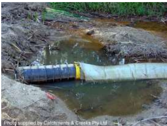
Filter tube outlet on a Type 2 sediment trap
