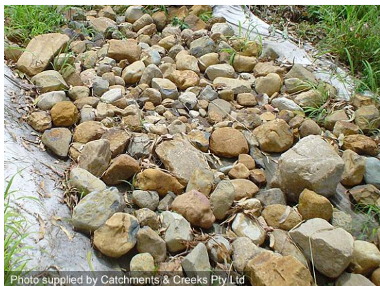
Rock-lined drainage channel
