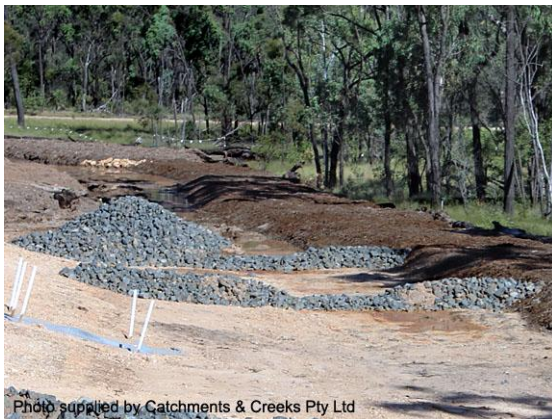
Velocity control check dams
