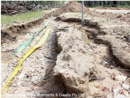
Storm damage to pipe trench
