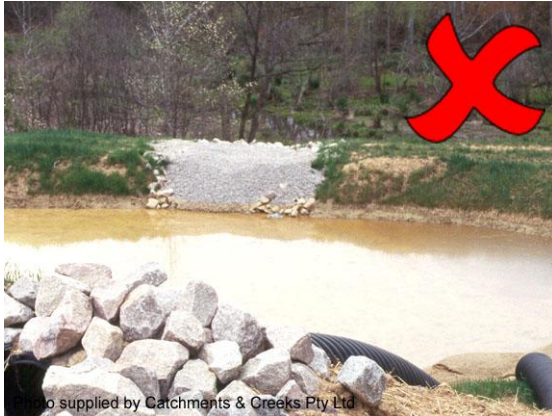
Poorly defined spillway crest
