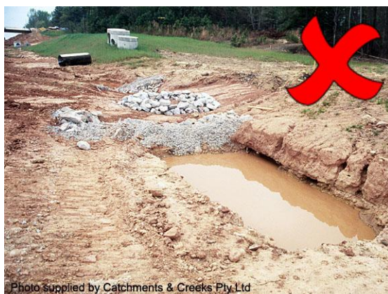
Sediment sump formed in dispersive soil
