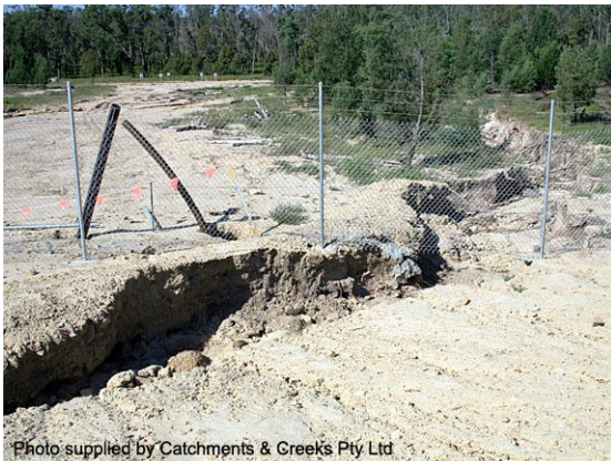
Gully erosion adjacent to pipe works
