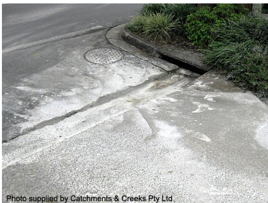
Deposition of cement wash-off on a road
