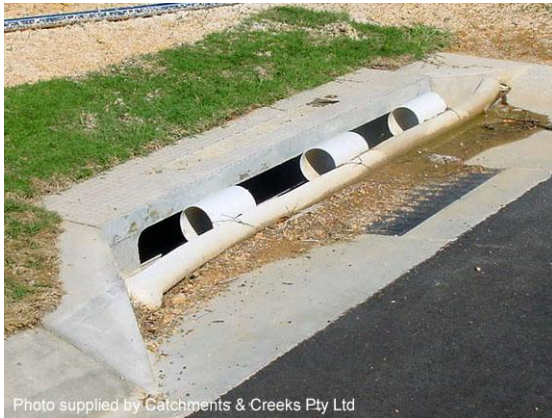
Sag inlet sediment trap
