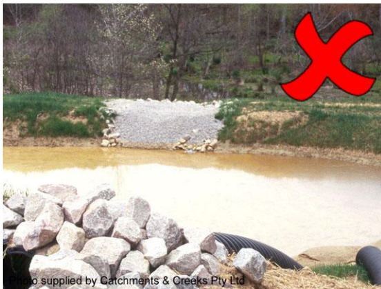
Poor sediment basin spillway design
