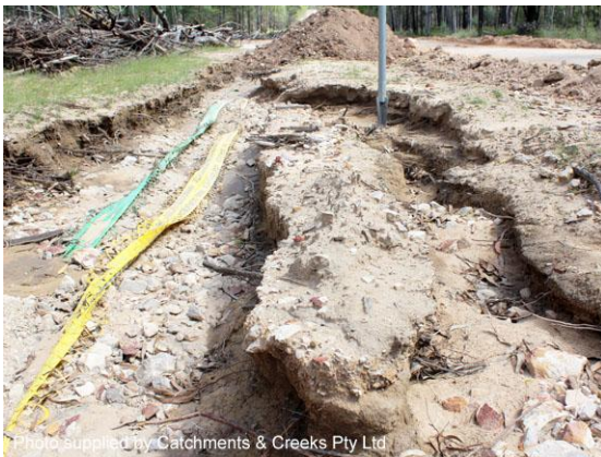
Erosion along a backfilled pipe trench
