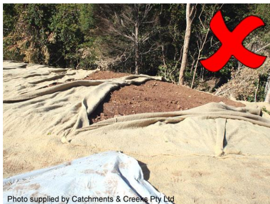
Blankets displaced by wind
