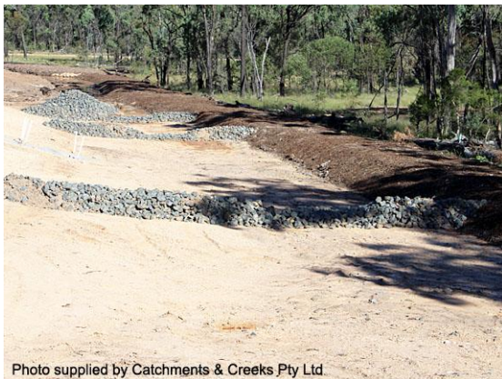
Velocity control check dams
