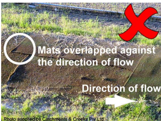
Mats overlapped in wrong direction
