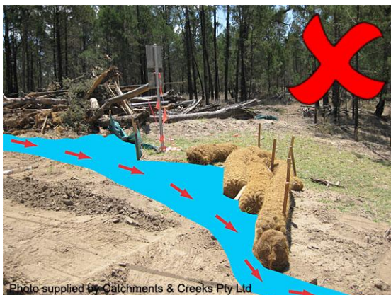
Stormwater runoff bypasses sediment trap
