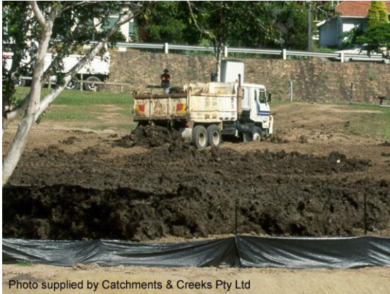
Truck bogged in wet soil
