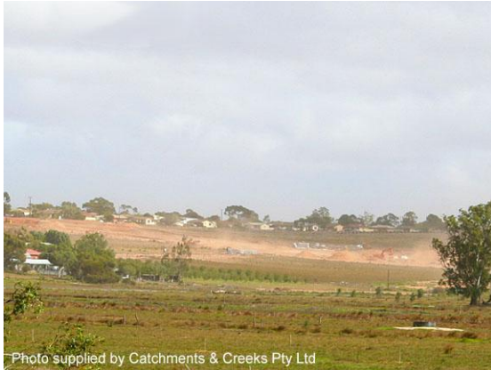
Construction site dust
