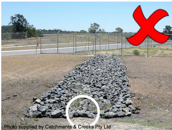
Inflow prevented from entering drain
