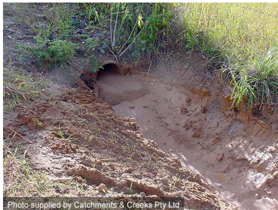
Deposition of sediment in a storm drain
