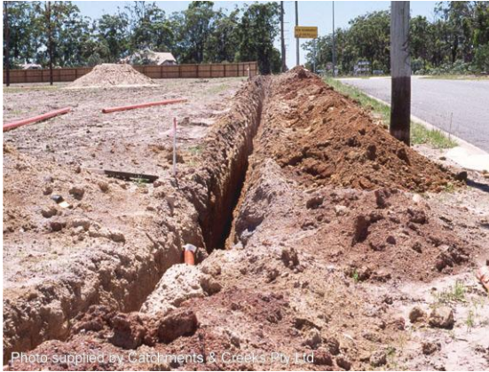
Domestic pipe installation
