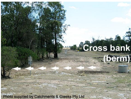
Cross drainage within pipeline RoW
