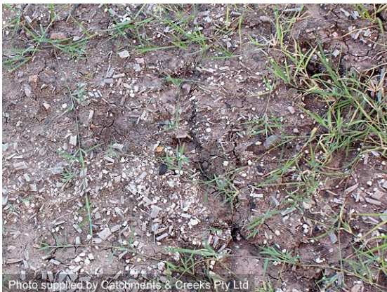
Embankment subject to sheet erosion
