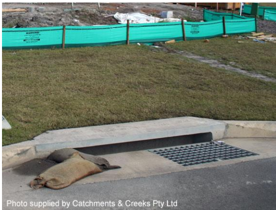
On-grade kerb inlet sediment trap
