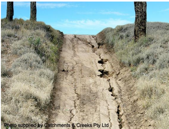
Rilling on a maintenance access track
