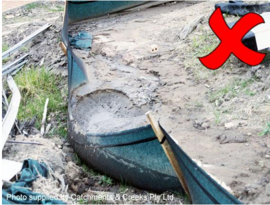
Sediment fence in need of maintenance
