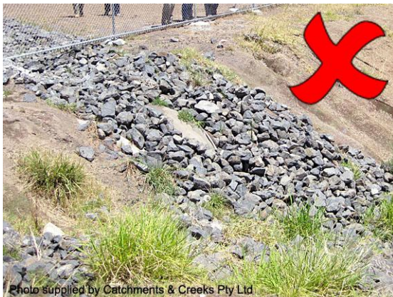
Rocks slipping down batter chute
