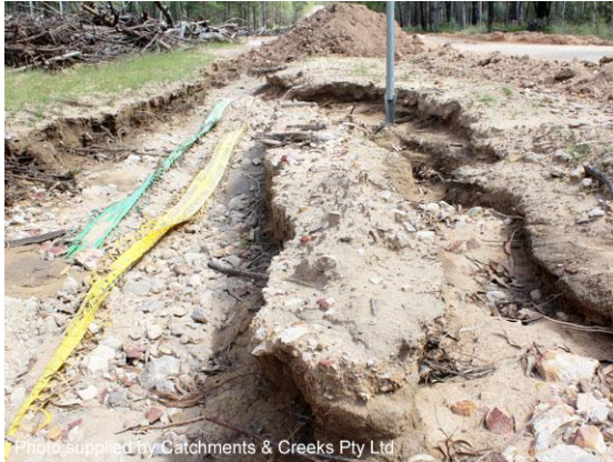
Storm damage to pipe trench
