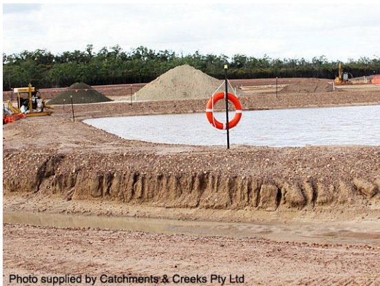
'Wet' type sediment basin
