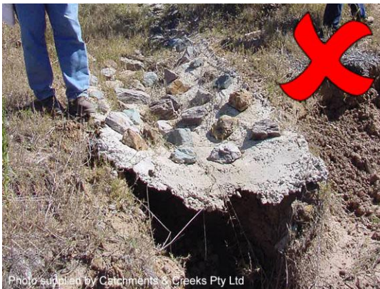
Tunnel erosion under concrete
