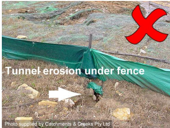
Storm damage to sediment fence
