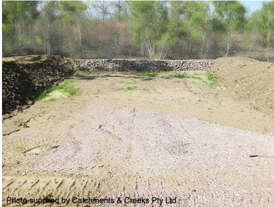
Rock filter dam
