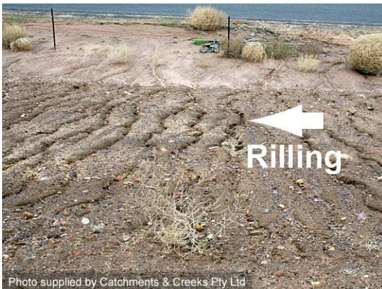
Rill erosion on an embankment
