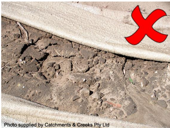
Inappropriate anchorage pegs
