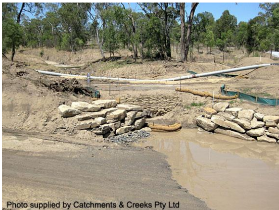
Pipeline crossing of a waterway
