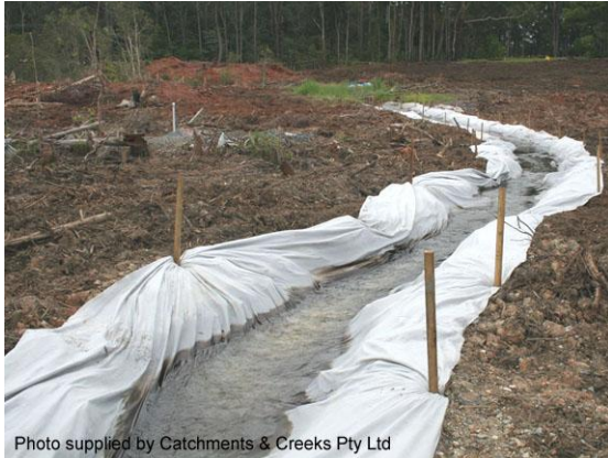
Clean water diversion drain
