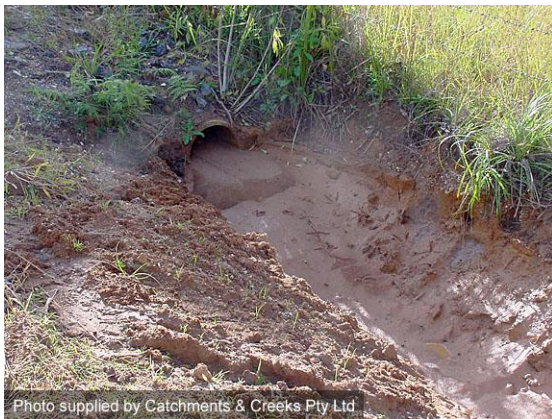
Sedimentation of drainage pipe
