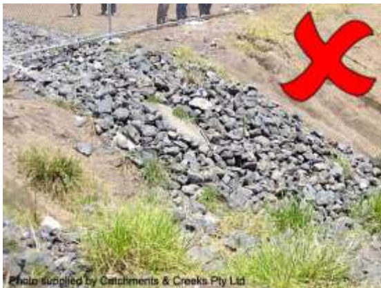
Rocks slipping down batter chute
