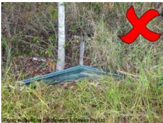
Sediment fence not removed after use
