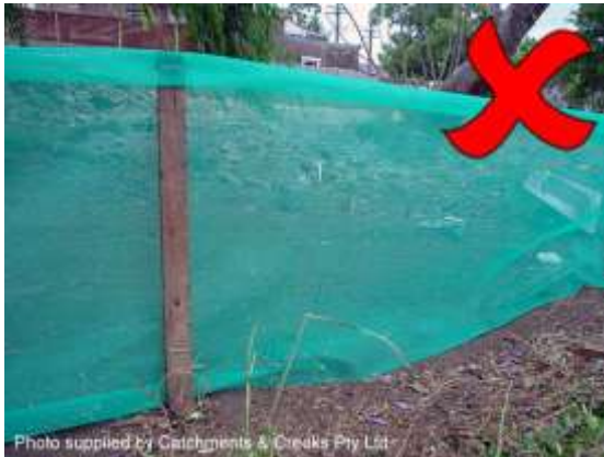
Inappropriate use of shade cloth
