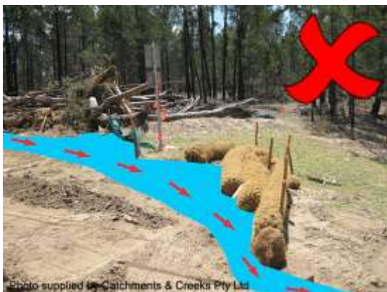
Stormwater runoff bypasses sediment trap
