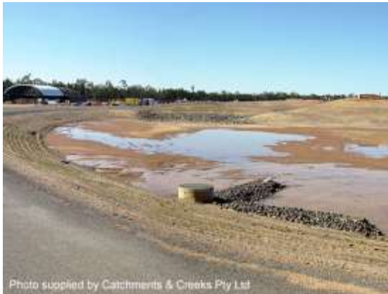
Sediment basin (Type-1)
