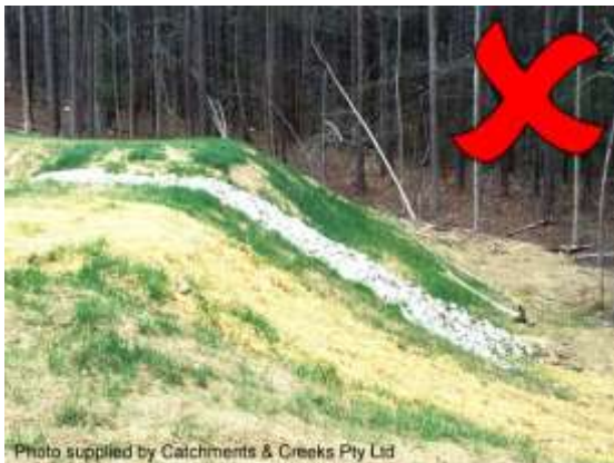
Insufficient scour protection at outlet
