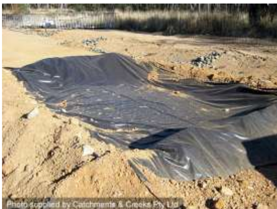
Concrete truck wash-out point
