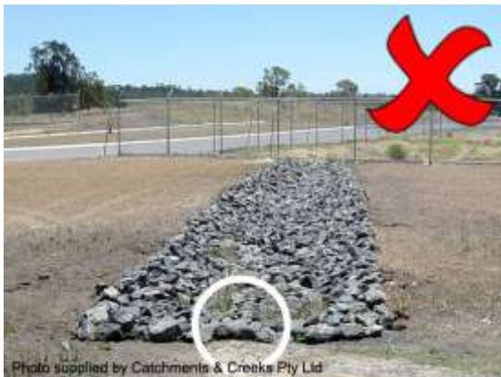
Inflow prevented from entering drain
