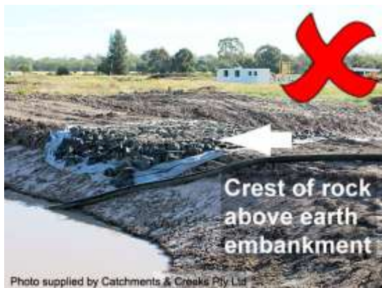
Inappropriate spillway crest profile
