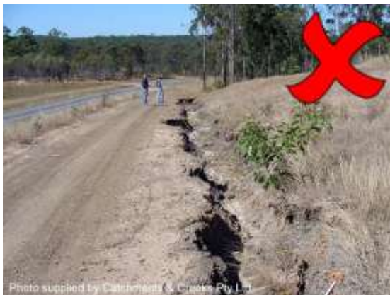
Catch drain cut into a dispersive soil
