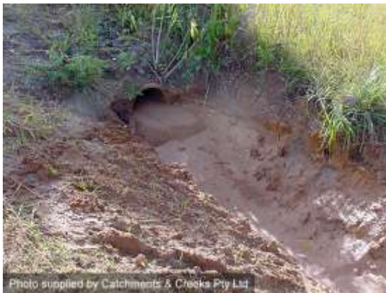
Sedimentation of drainage pipe
