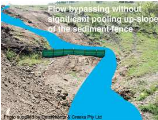
Sediment fence fails to capture sediment
