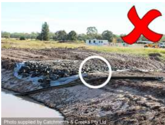
Rocks sit above the embankment height
