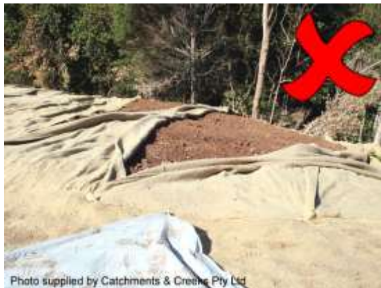
Blankets displaced by wind
