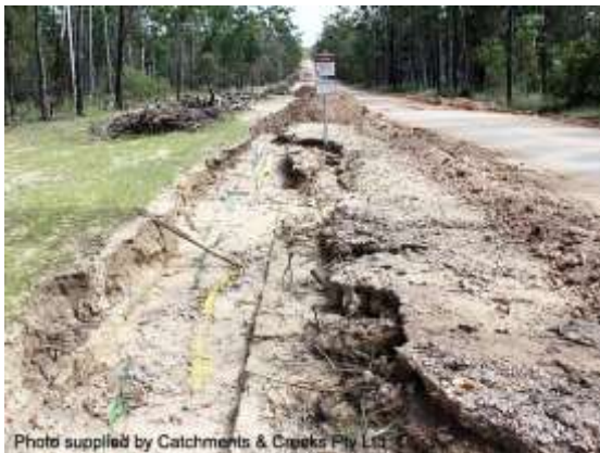
Erosion along a slaking soil trench
