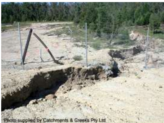
Gully erosion adjacent to pipe works
