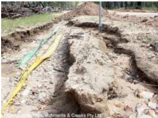
Storm damage to pipe trench
