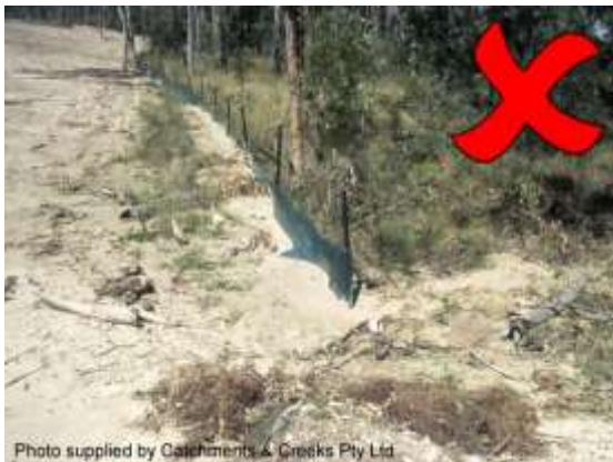
Fence not returned up-slope at end
