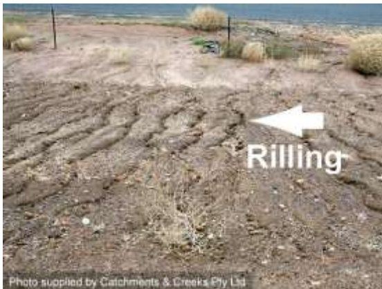
Rill erosion on an embankment
