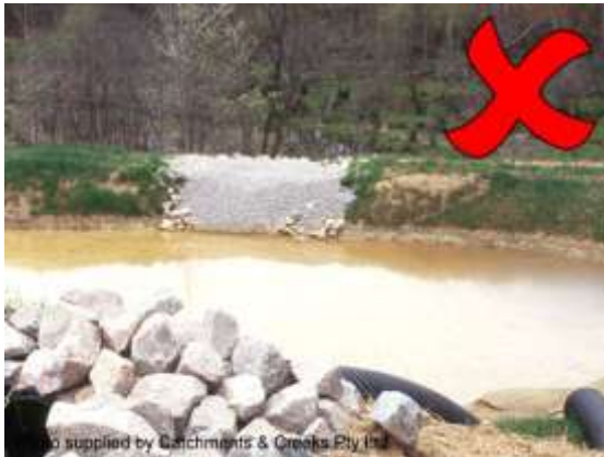
Poorly defined spillway crest
