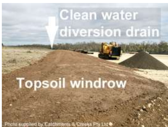
Topsoil windrow diversion drain
