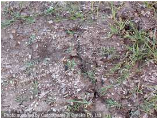
Embankment subject to sheet erosion
