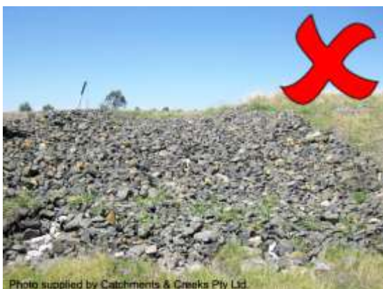
Inadequate rock size
