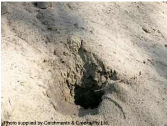
Inlet to tunnel erosion in pipe trench
