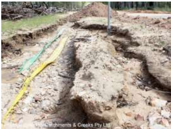
Erosion along a backfilled pipe trench
