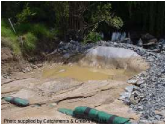
Rock filter dam (Type-2)
