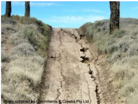
Rilling on a maintenance access track
