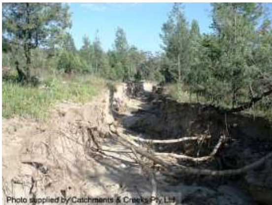
Recently formed gully erosion
