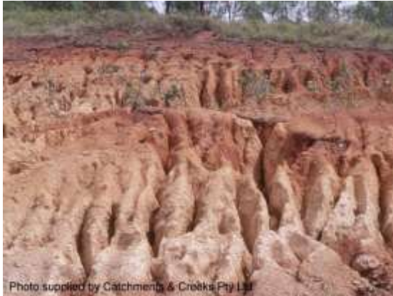
Erosion of a dispersive soil
