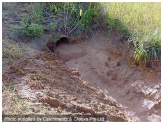
Deposition of sediment in a storm drain
