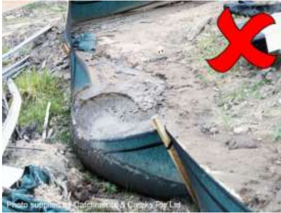
Sediment fence in need of maintenance
