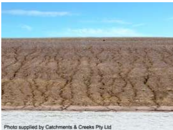
Severe rilling known as 'fluting'
