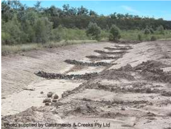
Check dam sediment trap
