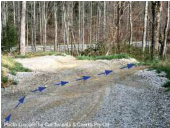
Cross bank drainage
