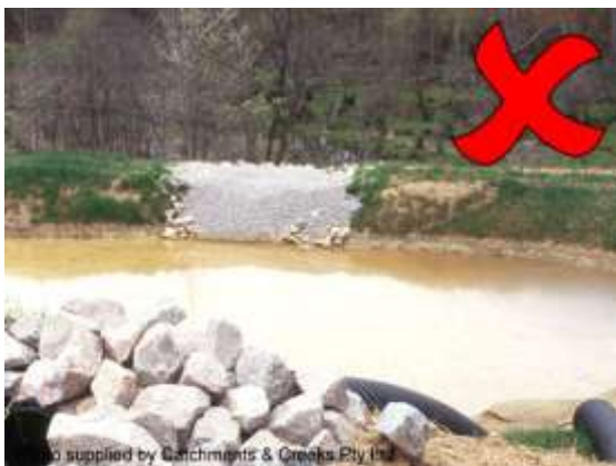
Poor sediment basin spillway design
