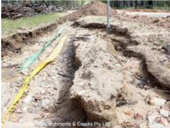
Storm damage to pipe trench
