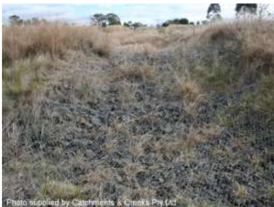
Rock mattress-lined basin spillway
