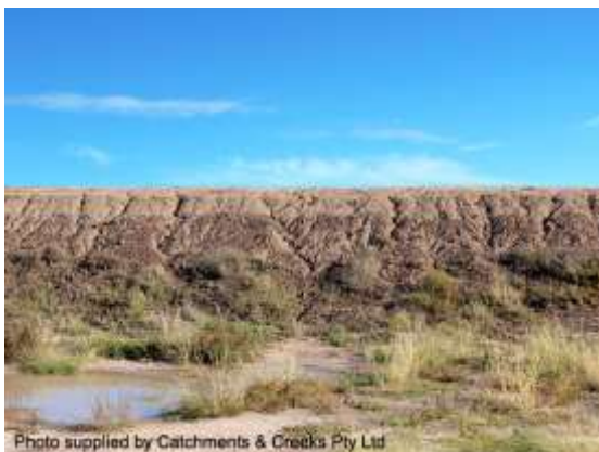
Rilling that extends to top of bank
