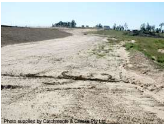
Rill erosion across an access track
