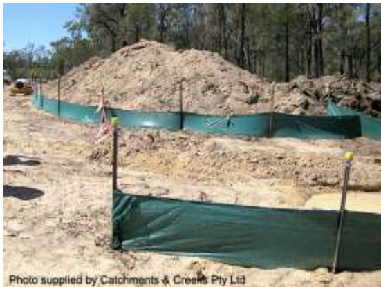
Sediment trap on pipeline RoW
