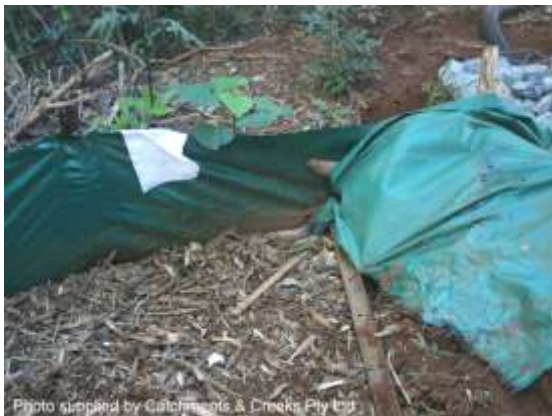
Damaged fence tagged for repair
