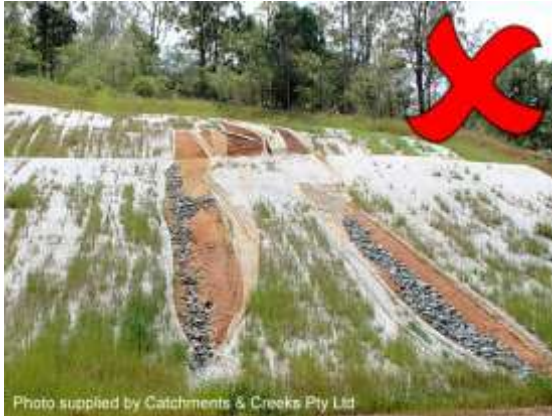
Blankets displaced by winds
