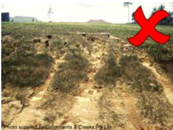
Erosion of recently seeded surface
