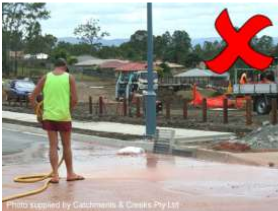
Poor maintenance practice
