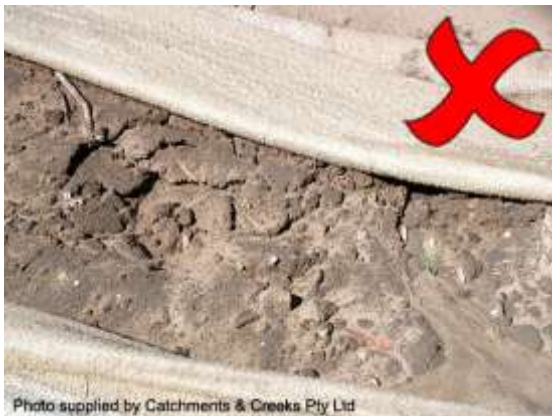
Inappropriate anchorage pegs
