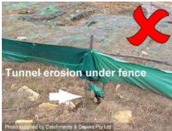
Storm damage to sediment fence
