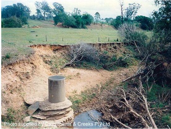
Bank erosion exposes sewer pipe
