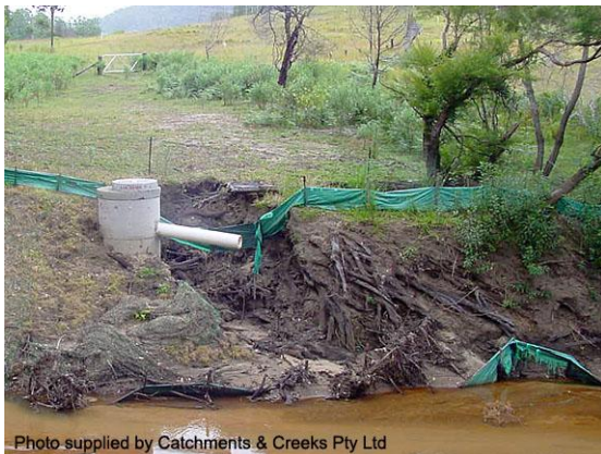
Bank erosion adjacent to an access pit
