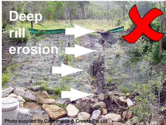
Failure of bank stabilisation works
