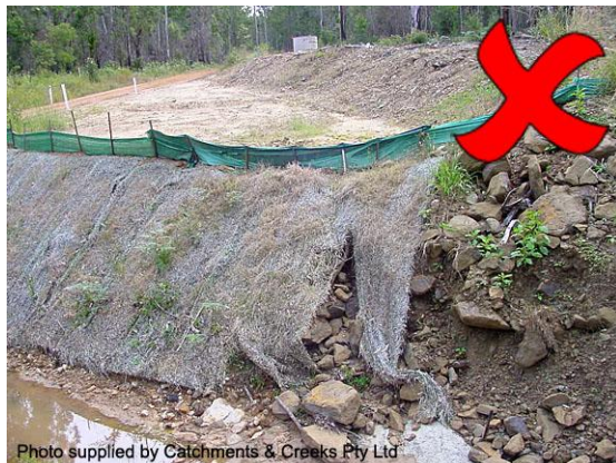
Bank erosion at a pipeline crossing
