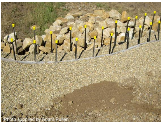
Sediment control weir
