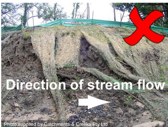
Failed erosion control mat
