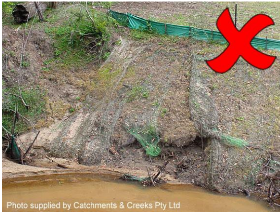
Erosion along toe of bank
