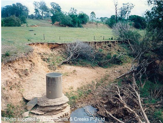
Bank erosion exposes sewer pipe chamber
