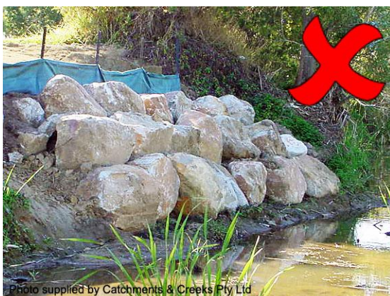
Poorly placed rocks on creek bank
