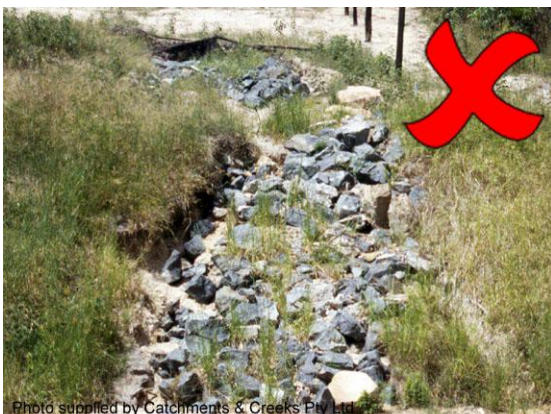
Rock placed on a dispersive soil bank
