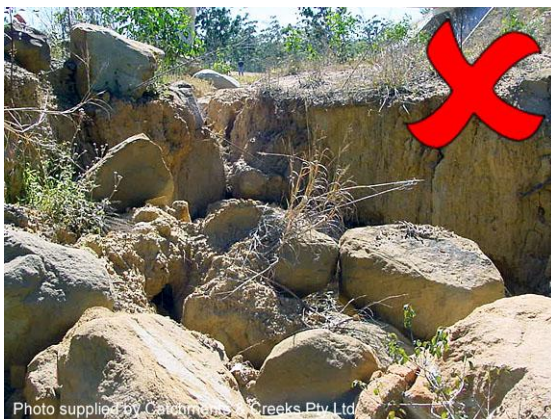
Collapsed dispersive soil bank
