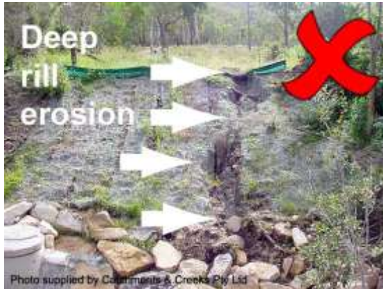
Failure of bank stabilisation works
