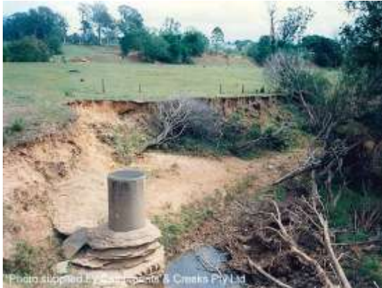
Bank erosion exposes sewer pipe chamber
