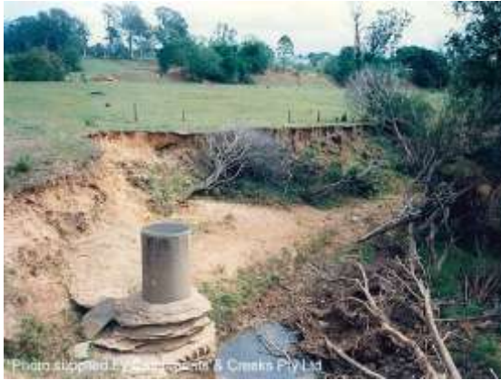
Bank erosion exposes sewer pipe
