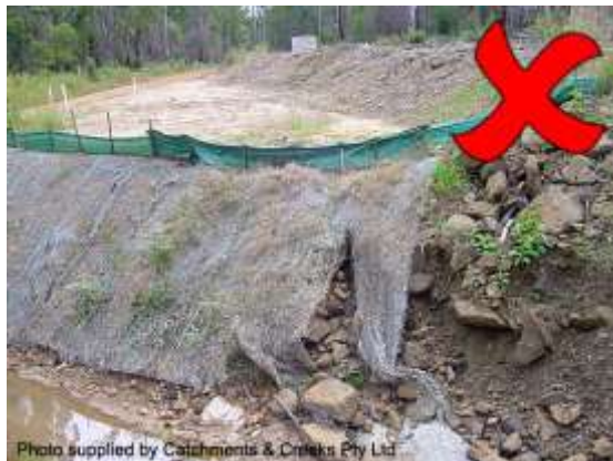
Bank erosion at a pipeline crossing
