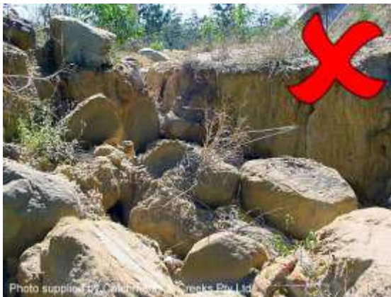
Collapsed dispersive soil bank
