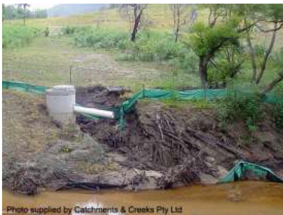
Bank erosion adjacent to an access pit
