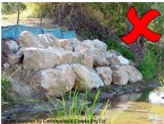
Poorly placed rocks on creek bank
