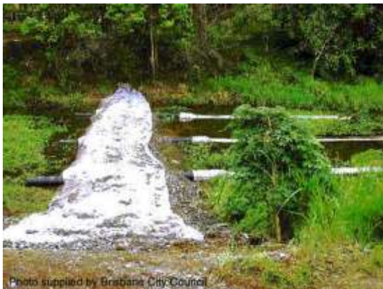
Rock filter dam with filter tubes
