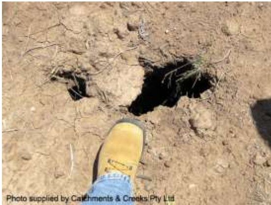
Tunnel erosion above pipeline
