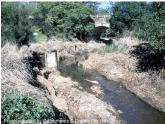
Bank erosion downstream of chamber
