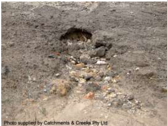
Outlet of above tunnel erosion
