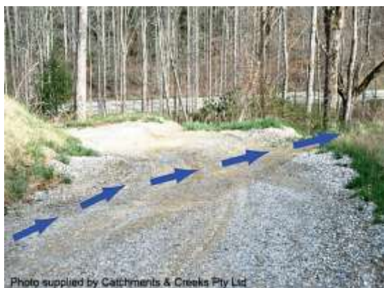
Flows diverted off access track
