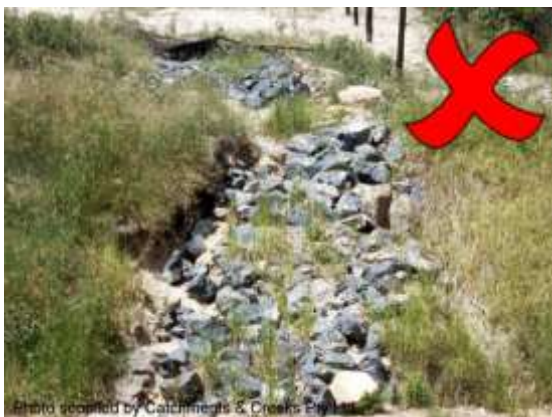
Rock placed on a dispersive soil bank
