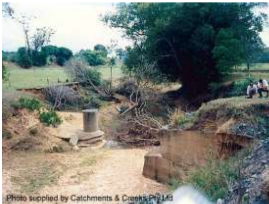
Pipeline exposed by migrating waterway
