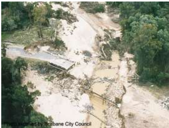
Flood damage to bridge & buried pipes
