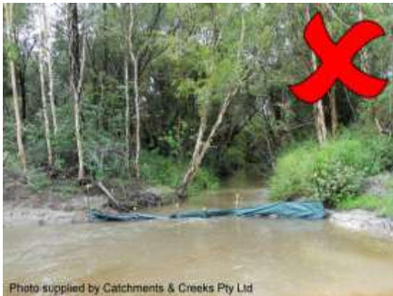
Inappropriate instream sediment control
