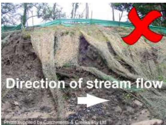
Failed erosion control mat
