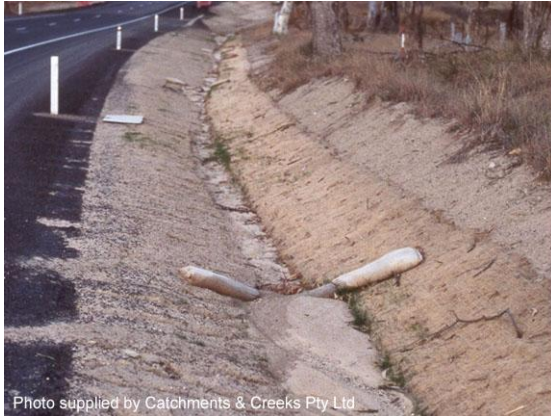
Check dam sediment trap
