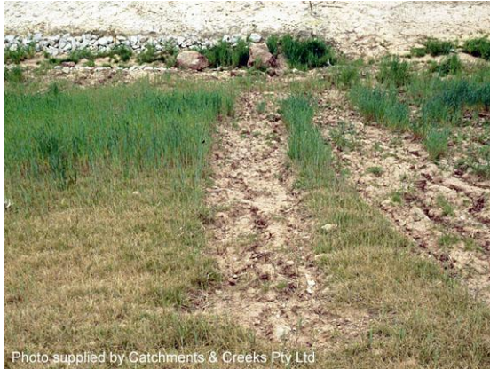
Rilling on a newly seeded batter
