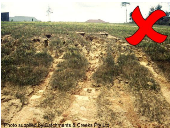
Erosion of recently seeded surface
