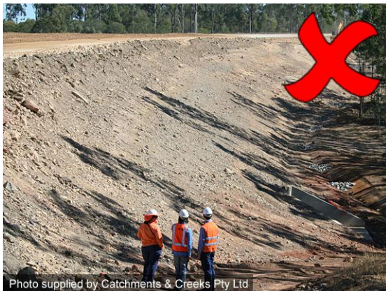
Batter without appropriate erosion control
