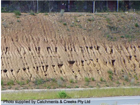
Severe rilling within a dispersive soil
