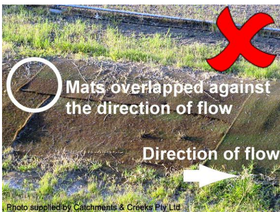
Mats overlapped in wrong direction
