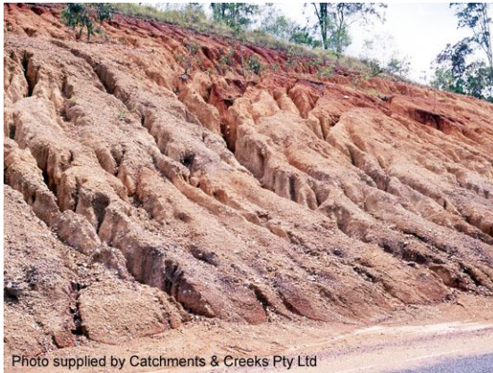
Condition prior to bank repair (1997)
