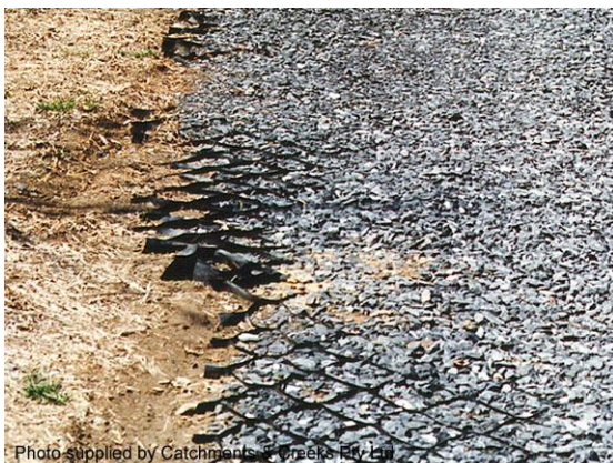
Gravelled car park
