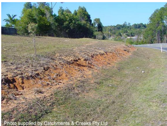
Loss of vegetation from the road batter
