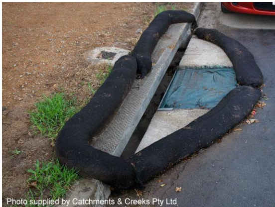
Kerb inlet protection (supplementary)
