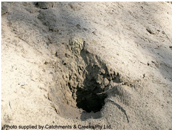
Inlet to tunnel erosion in pipe trench
