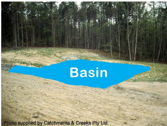
Roadside sediment basin
