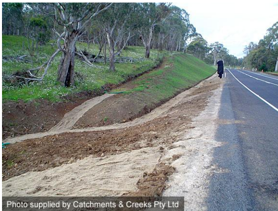
Catch drain and table drain
