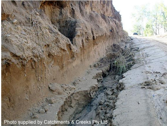
Deep rilling within a sandy soil
