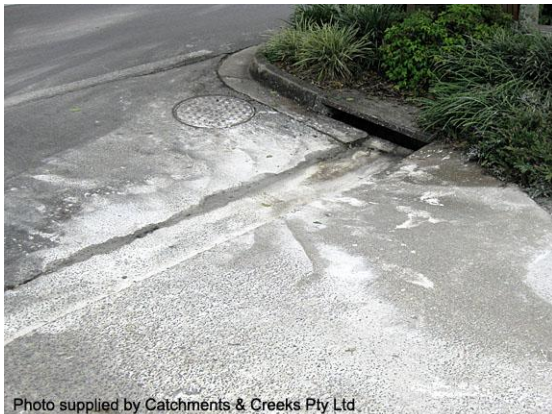
Deposition of cement wash-off on a road
