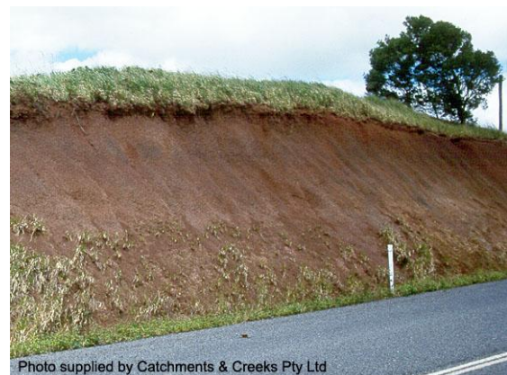
Eroded road batter
