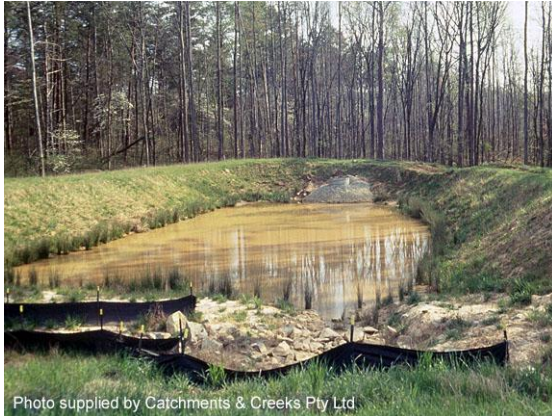
Sediment basin (Type-1)
