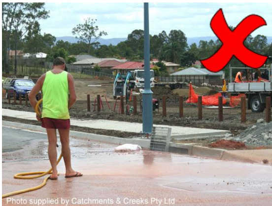
Poor maintenance practice
