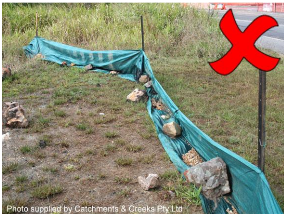
Toe of fabric incorrectly anchored
