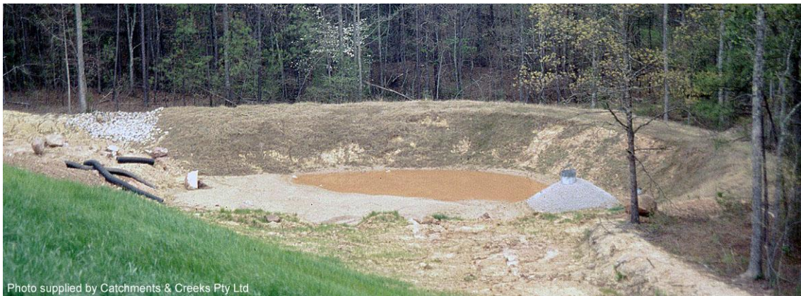
Type-C sediment basin with riser pipe outlet (1995)
