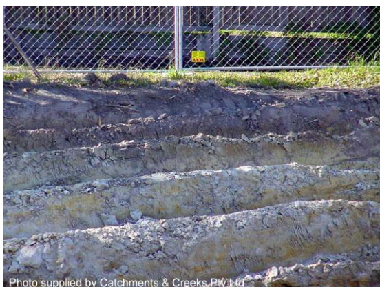
Stair-stepping of steep batter
