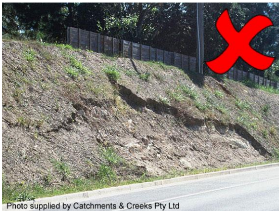
Slippage of topsoil from steep batter
