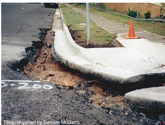
Storm damage to road works
