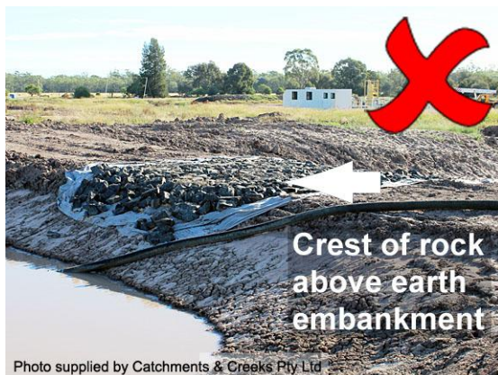
Inappropriate spillway crest profile
