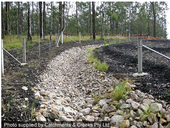
Rock-lined catch drain
