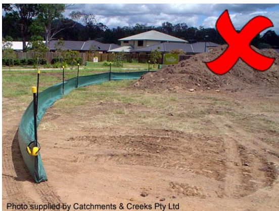
Post placed on wrong side of fence
