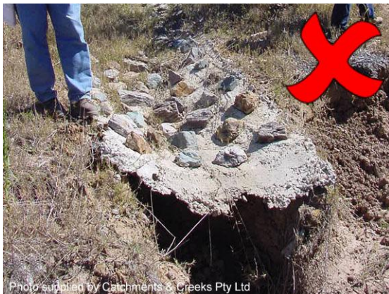
Tunnel erosion under concrete
