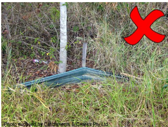
Sediment fence not removed after use
