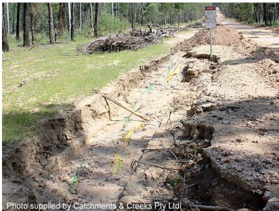
Erosion of backfilled service trench
