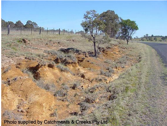
Erosion of a dispersive soil
