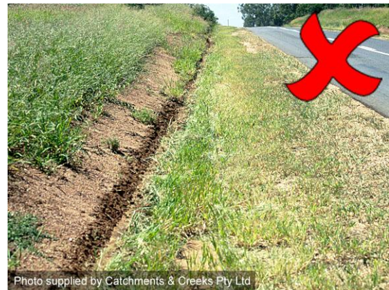
Mechanical disturbance of batter toe
