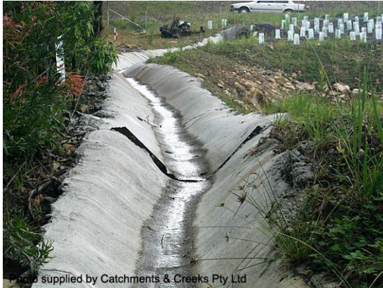
Concrete-lined catch drain
