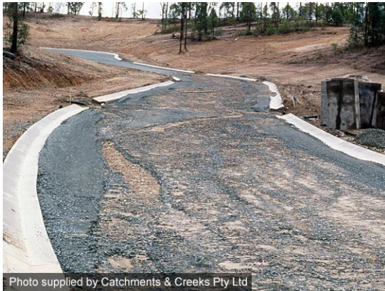
Storm damage to pavement road base
