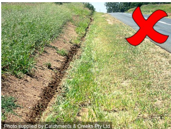
Scour damage to batter toe
