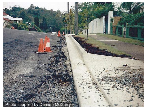
Storm damage to road works
