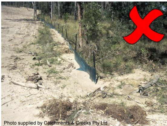
Fence not returned up-slope at end
