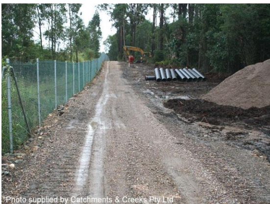
Unsealed construction access road
