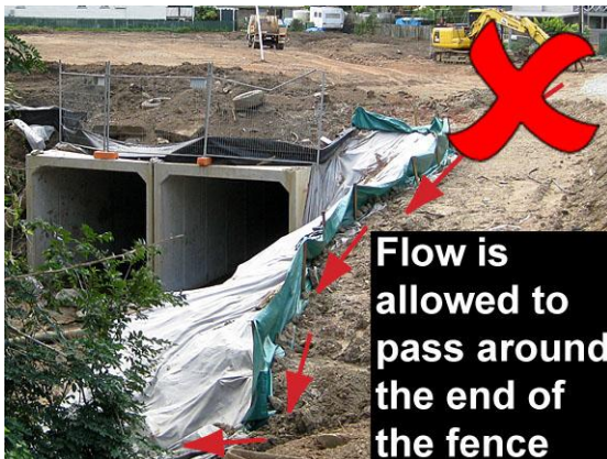
Sediment fence fails to capture sediment
