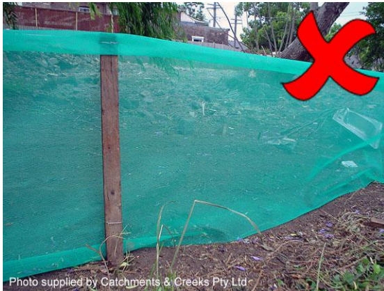
Inappropriate use of shade cloth
