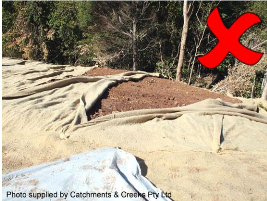
Blankets displaced by winds
