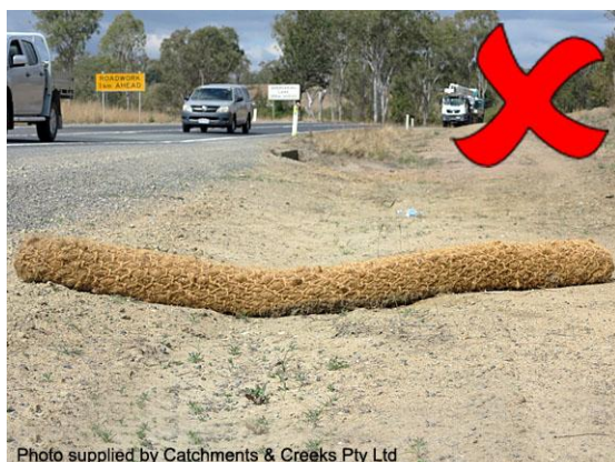
Geo log not adequately staked
