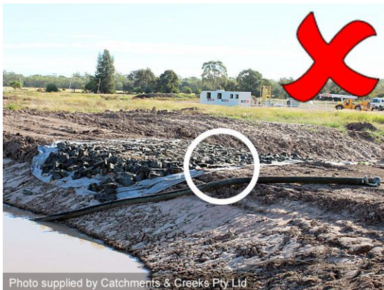
Rocks sit above the embankment height
