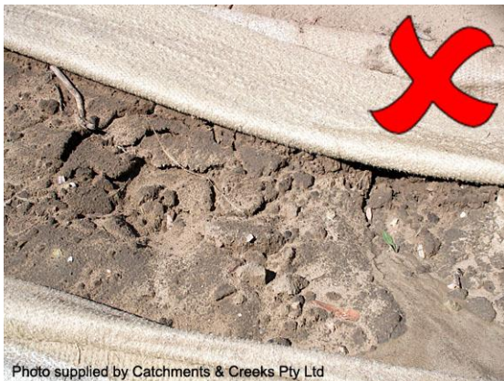
Inappropriate anchorage pegs
