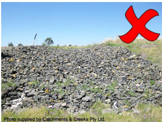
Inadequate rock size
