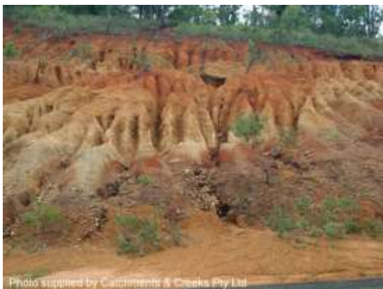
Erosion of an exposed dispersive soil
