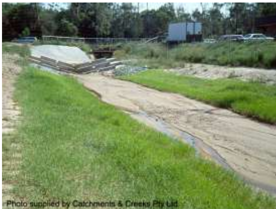
Deposition of sediment in a storm drain
