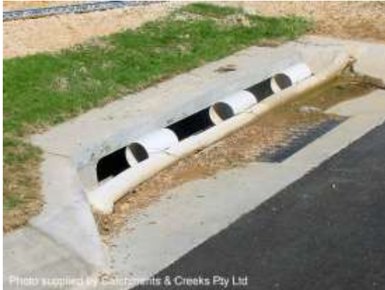
Sag inlet sediment trap
