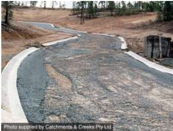
Storm damage to pavement road base
