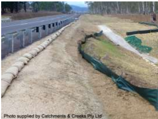
Sandbags used to divert road runoff
