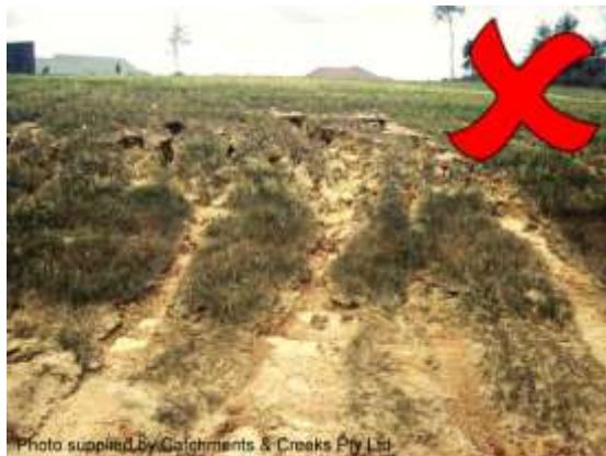
Failed revegetation of a dispersive soil
