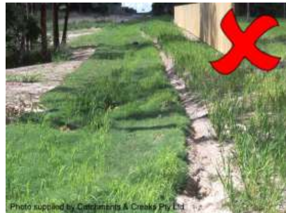
Rilling along the edge of turf
