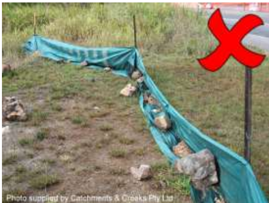
Toe of fabric incorrectly anchored
