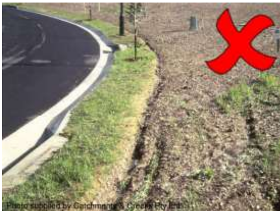
Rilling along the edge of turf
