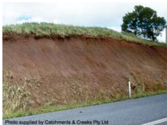
Eroded road batter
