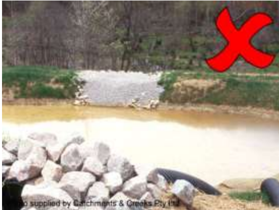
Poorly defined spillway crest
