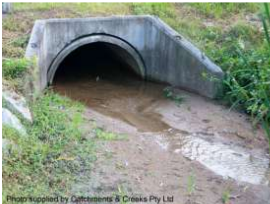
Sedimentation of drainage pipe
