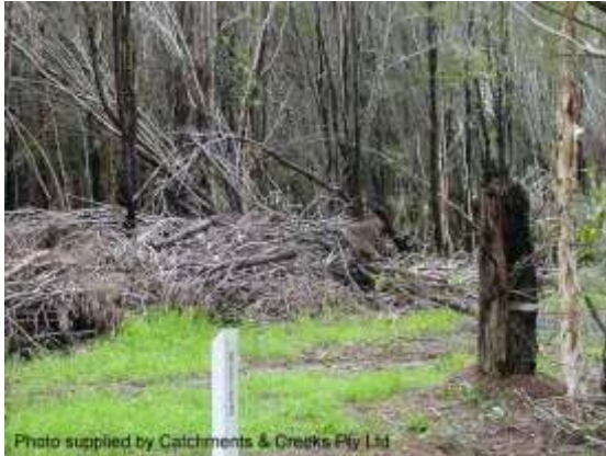
Brushwood barrier sediment trap
