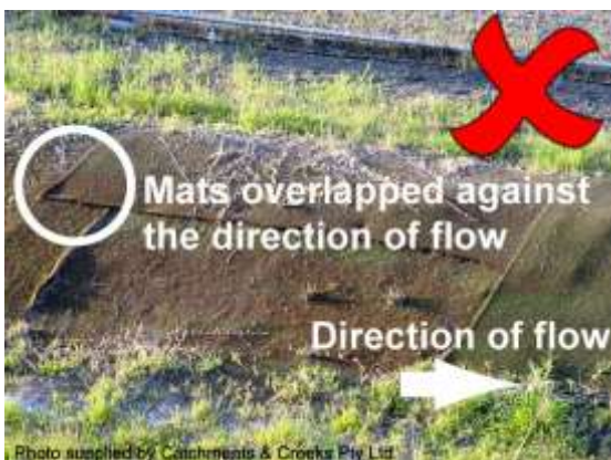
Mats overlapped in wrong direction
