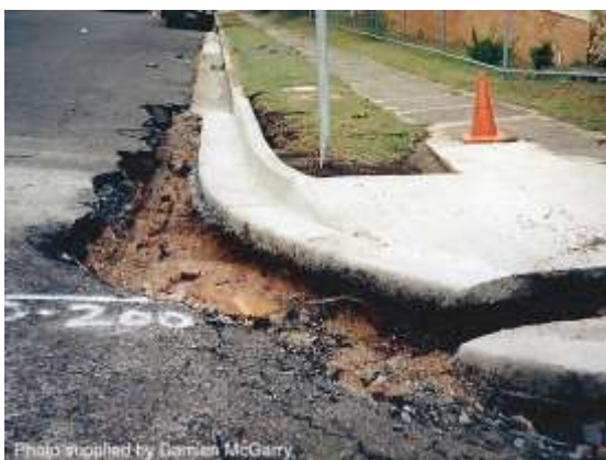
Storm damage to road works
