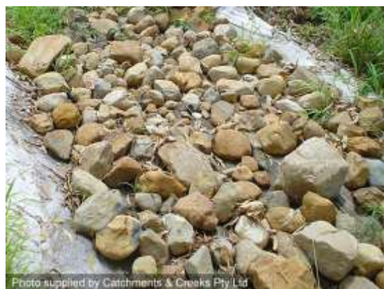
Rock-lined drainage channel
