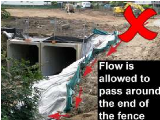
Sediment fence fails to capture sediment
