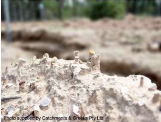
Evidence of raindrop impact erosion
