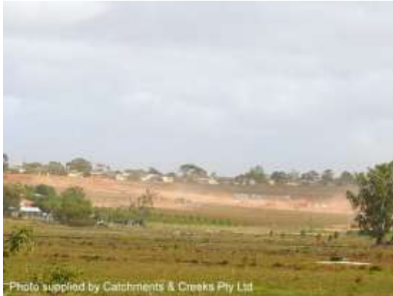
Construction site dust
