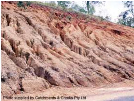
Condition prior to bank repair (1997)
