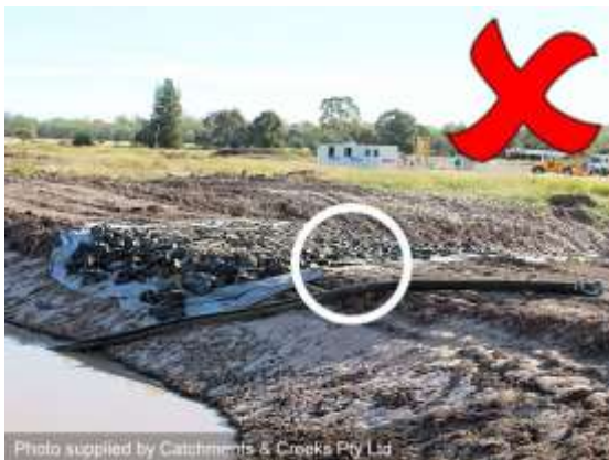
Rocks sit above the embankment height
