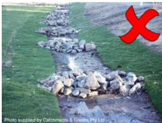
Flows forced to pass around check dams
