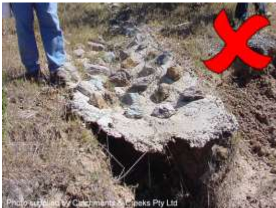
Tunnel erosion under concrete
