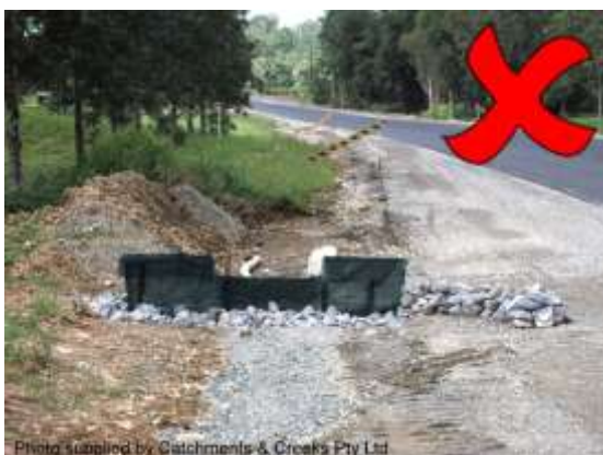
Common sense gone missing!
