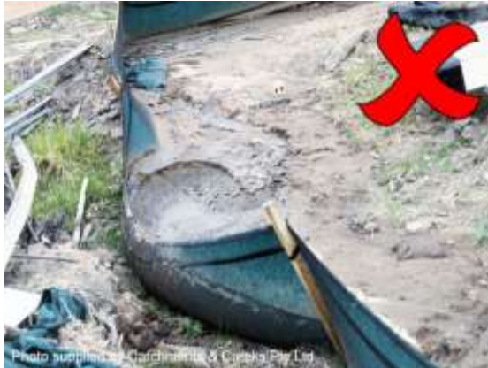
Sediment fence in need of maintenance
