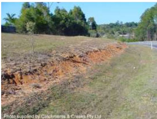
Loss of vegetation from the road batter
