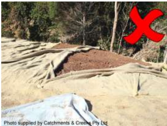
Blankets displaced by wind
