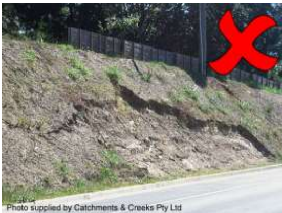
Slippage of topsoil from steep batter
