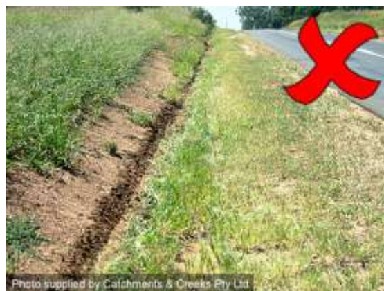
Mechanical disturbance of batter toe
