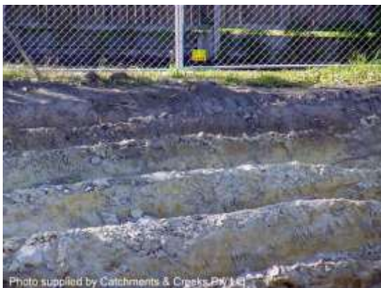
Stair-stepping of steep batter
