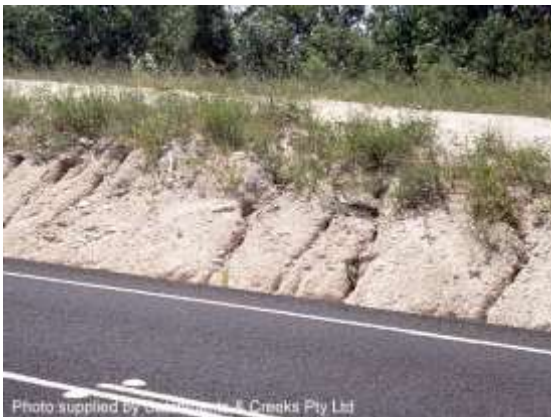
Rill erosion on a cut batter
