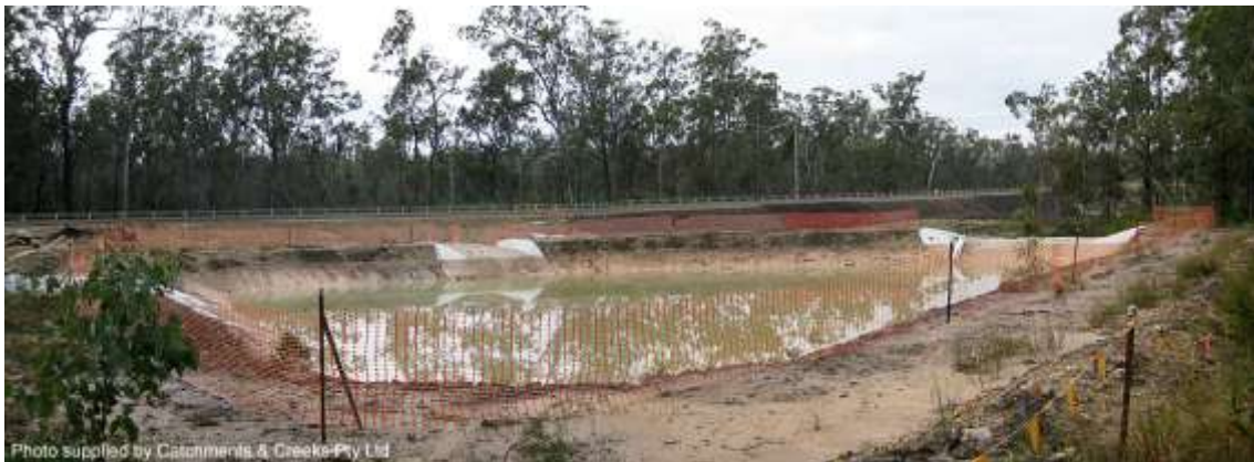
Type-C sediment basin with siphon pipe decant system (2017)
