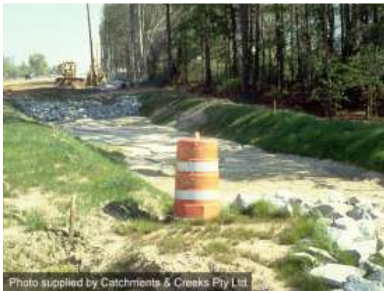
Rock filter dam
