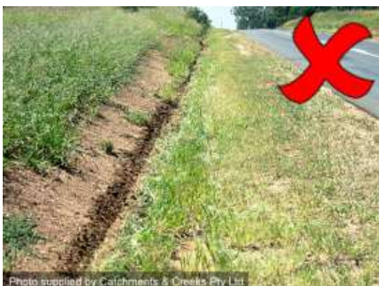
Scour damage to batter toe
