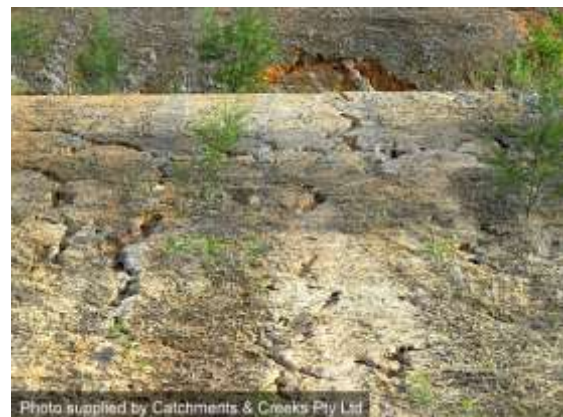
Evidence of ongoing rill erosion (2013)
