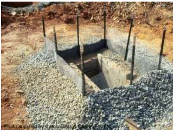
Mesh & aggregate drop inlet protection
