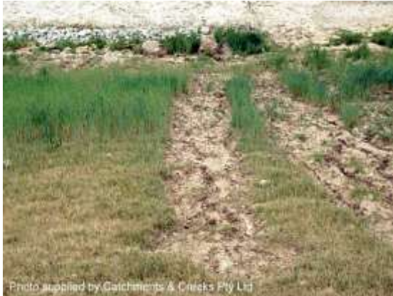
Rilling on a newly seeded batter
