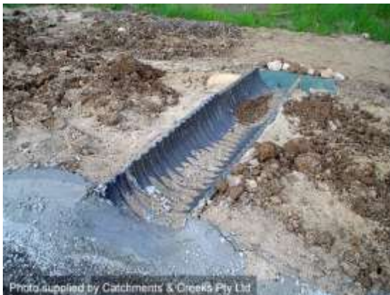
Temporary half-pipe batter chute
