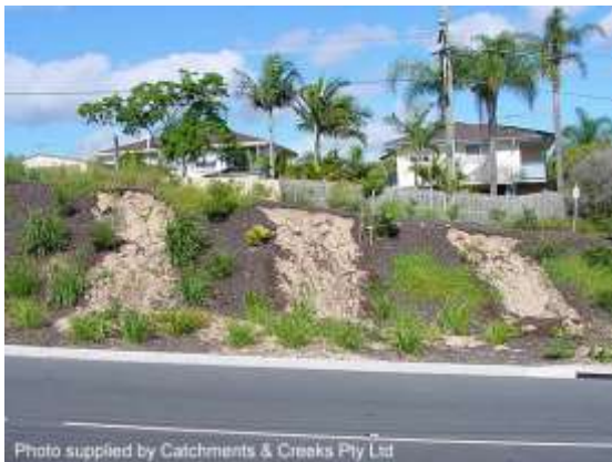
Storm damage to road batter
