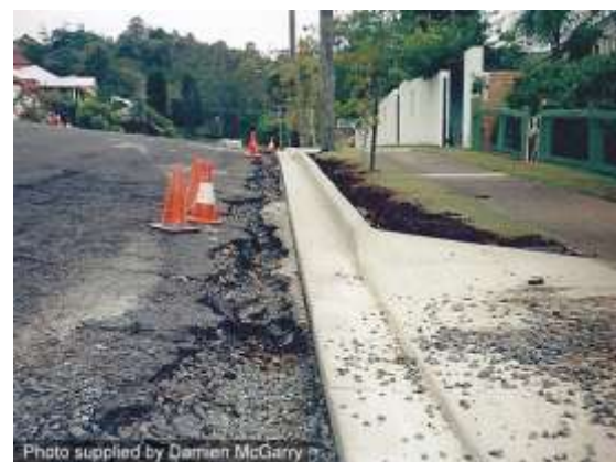
Storm damage to road works
