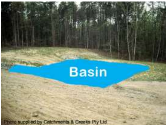
Roadside sediment basin
