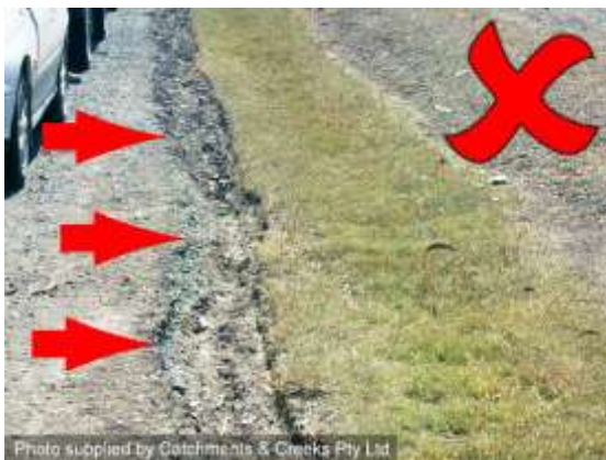
Rilling along the edge of turf
