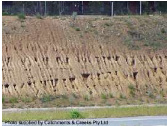
Severe rilling within a dispersive soil
