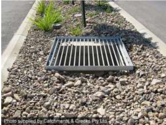
Field inlet located within median strip
