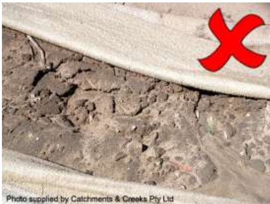
Inappropriate anchorage pegs
