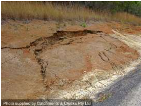
Bank slumping on a cut batter
