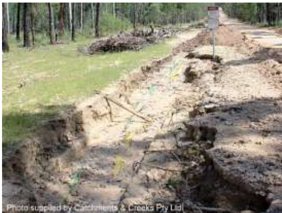
Erosion of backfilled service trench
