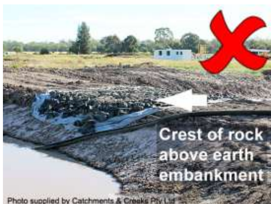
Inappropriate spillway crest profile
