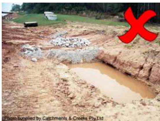
Sediment sump formed in dispersive soil
