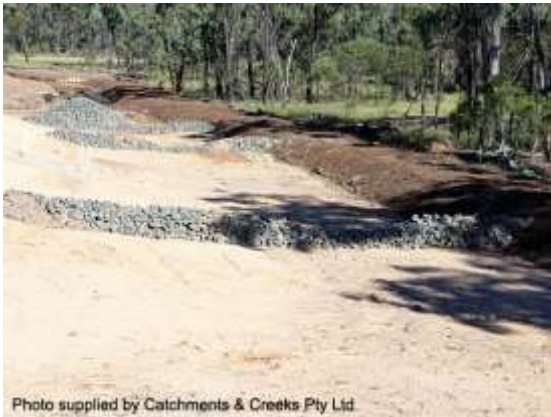
Velocity control check dams
