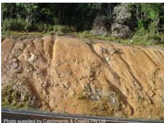
Rilling that extends to top of bank
