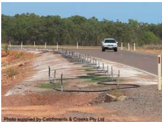
Temporary irrigation system
