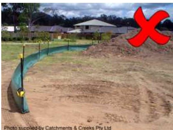
Post placed on wrong side of fence
