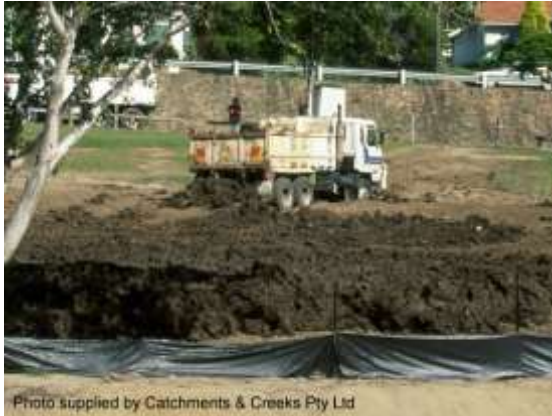
Truck bogged in wet soil
