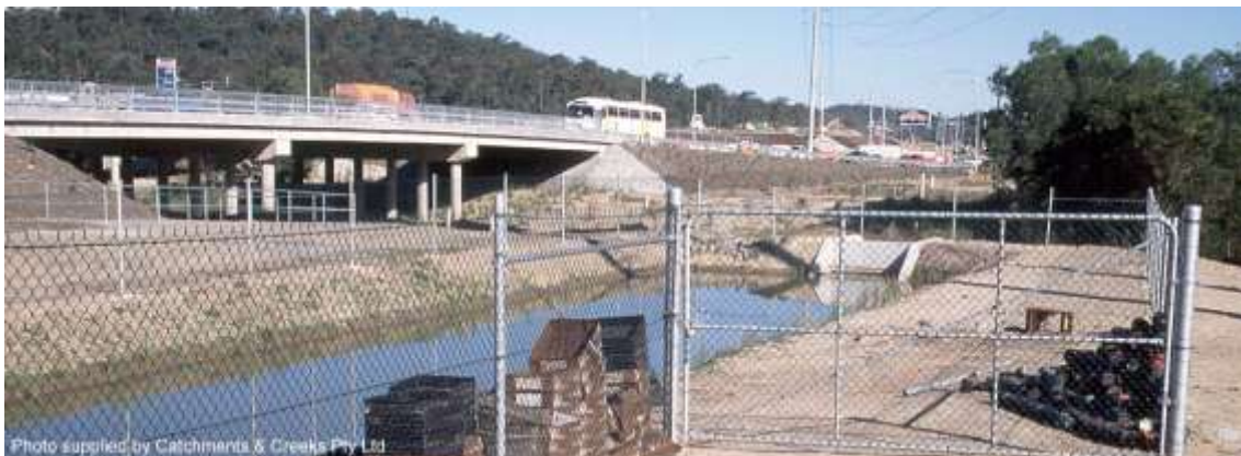
Type-D sediment basin which is retained for permanent stormwater treatment (1999)
