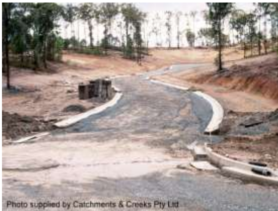
Storm damage to road works
