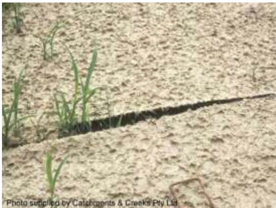
Soil erosion occurring under blanket
