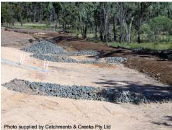
Velocity control check dams
