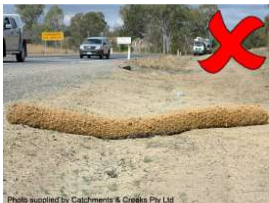
Geo log not adequately staked
