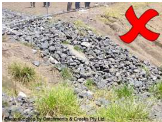
Rocks slipping down batter chute
