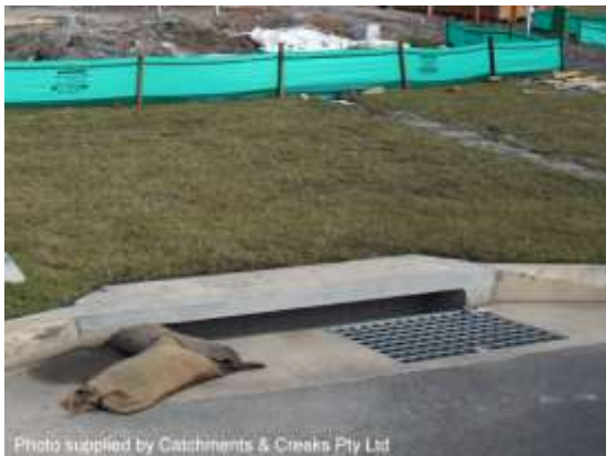
On-grade kerb inlet sediment trap
