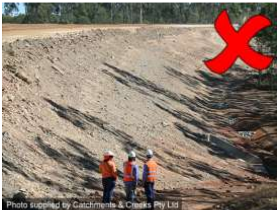
Batter without appropriate erosion control
