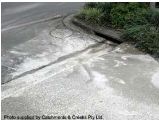
Deposition of cement wash-off on a road
