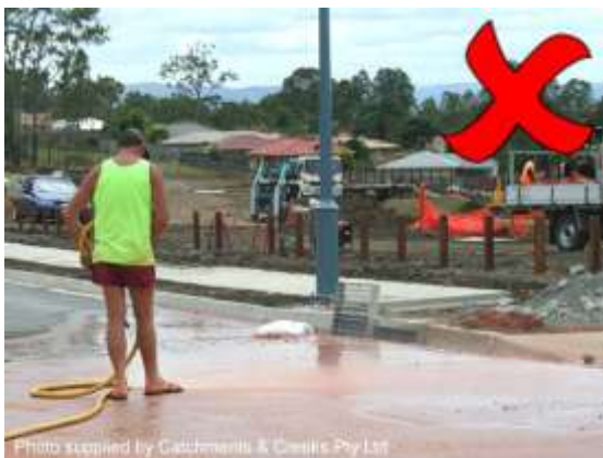
Poor maintenance practice
