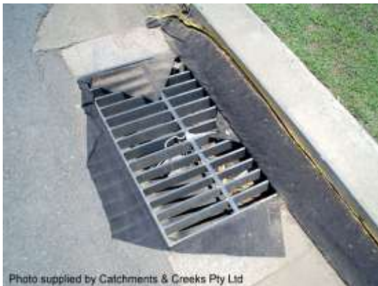
Gully bag sediment trap
