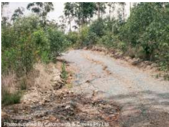
Damage to construction access road
