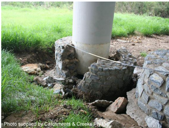
Flood damage to bridge pier
