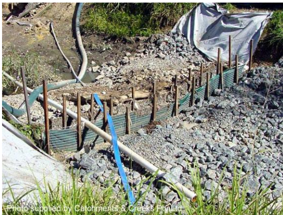
Instream sediment weir
