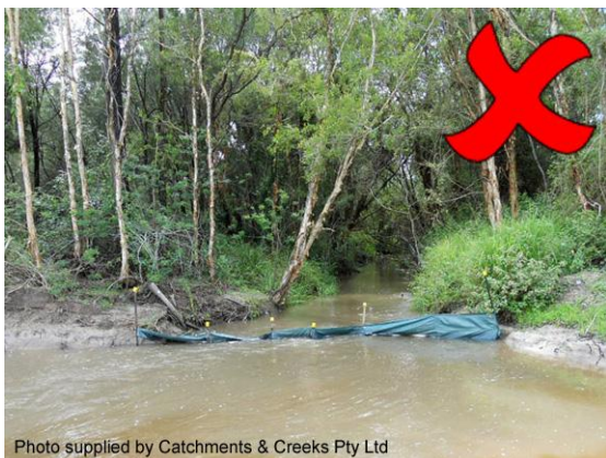
Inappropriate instream sediment control
