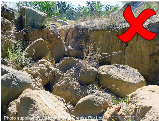
Collapsed dispersive soil bank
