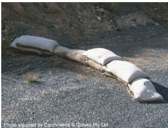
Check dam sediment trap
