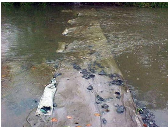
Elevated stream flows at work site
