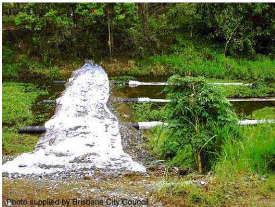
Rock filter dam with filter tubes
