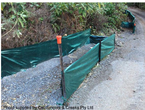
U-shaped sediment trap on mild slope
