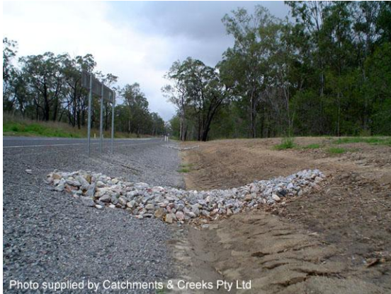
Velocity control check dam
