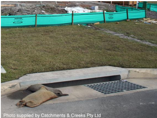
'On-grade' kerb inlet sediment trap
