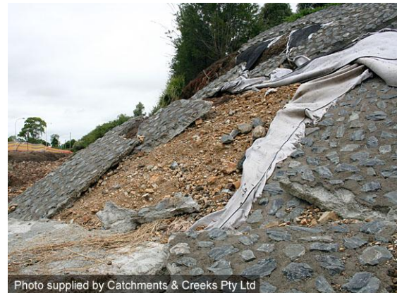
Failed stone pitching (same bridge)
