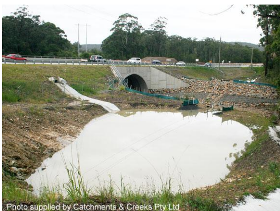
Stormwater treatment pond (2009)
