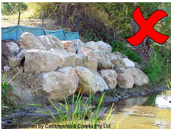
Poorly placed rocks on creek bank
