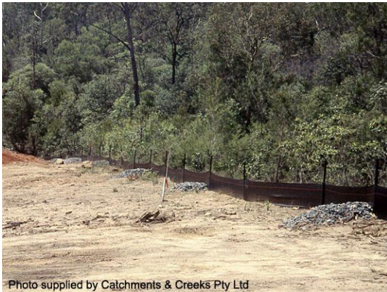
Check dams adjacent to a sediment fence
