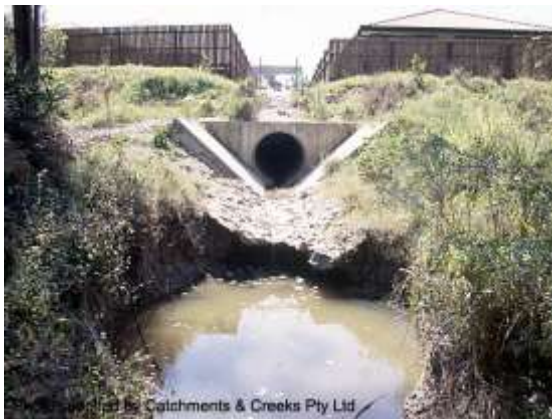
Urban stormwater pipe drainage line
