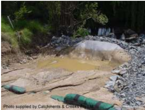
Rock filter dam (Type-2 sediment trap)
