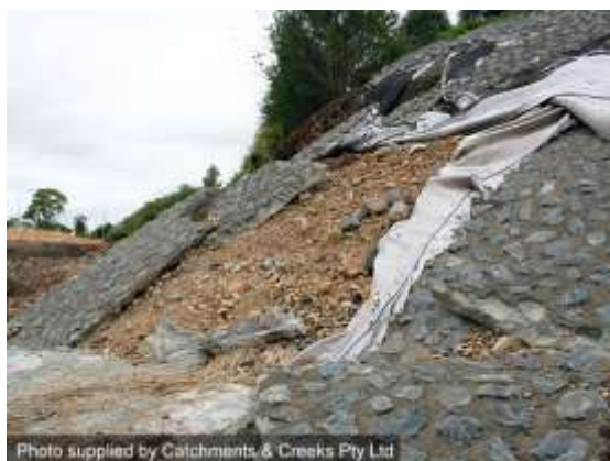
Failed stone pitching (same bridge)
