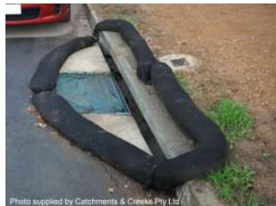
'Sag' kerb inlet sediment trap
