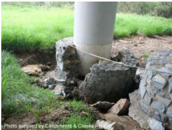
Flood damage to bridge pier
