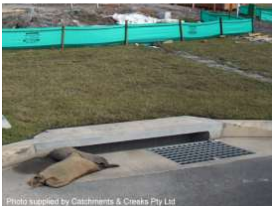
'On-grade' kerb inlet sediment trap
