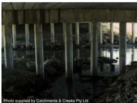
Poor light conditions under a bridge
