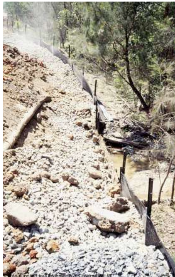
Spill-through weir & aggregate filter
