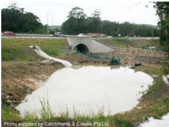
Stormwater treatment pond (2009)
