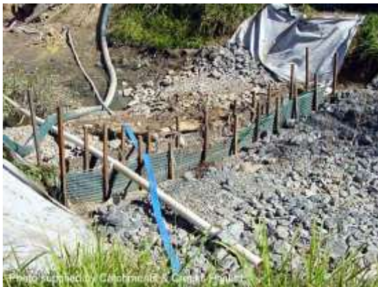
Instream sediment weir
