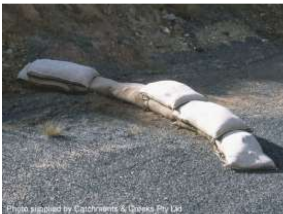
Check dam sediment trap
