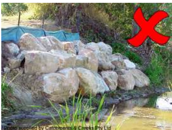
Poorly placed rocks on creek bank
