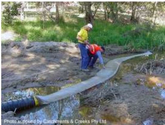
Instream sediment control system
