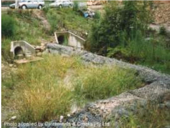
Roadside bio-retention system
