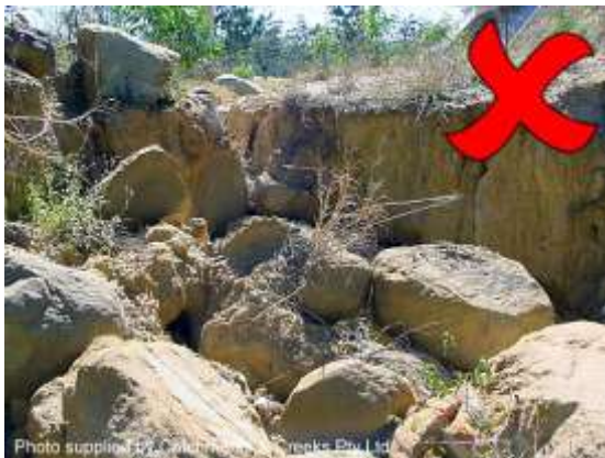
Collapsed dispersive soil bank
