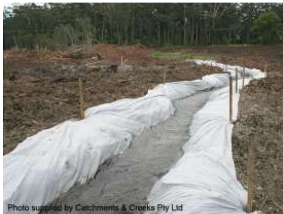
Clean water cross-drainage system
