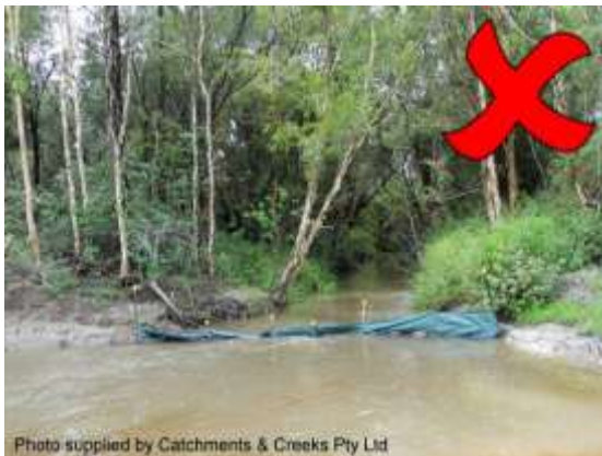
Inappropriate instream sediment control
