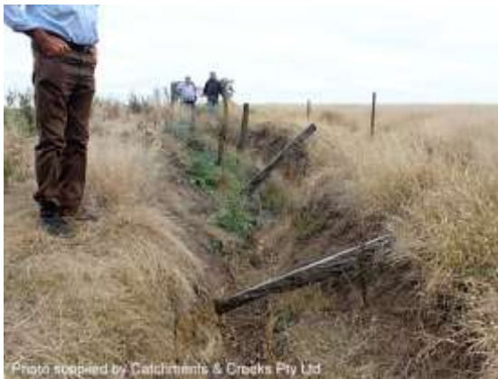
Gully erosion along a fence line (Qld)
