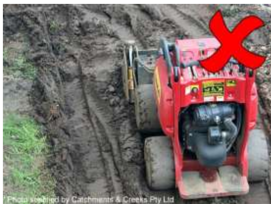
Excess working of saturated soils
