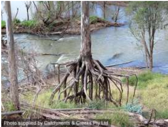
Exposure of roots by severe bank erosion
