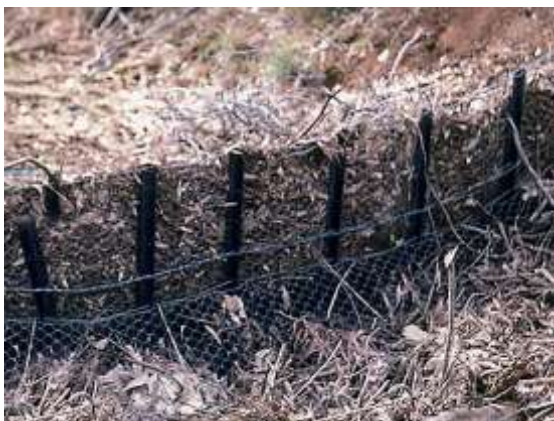
Leaky weir (NSW)
